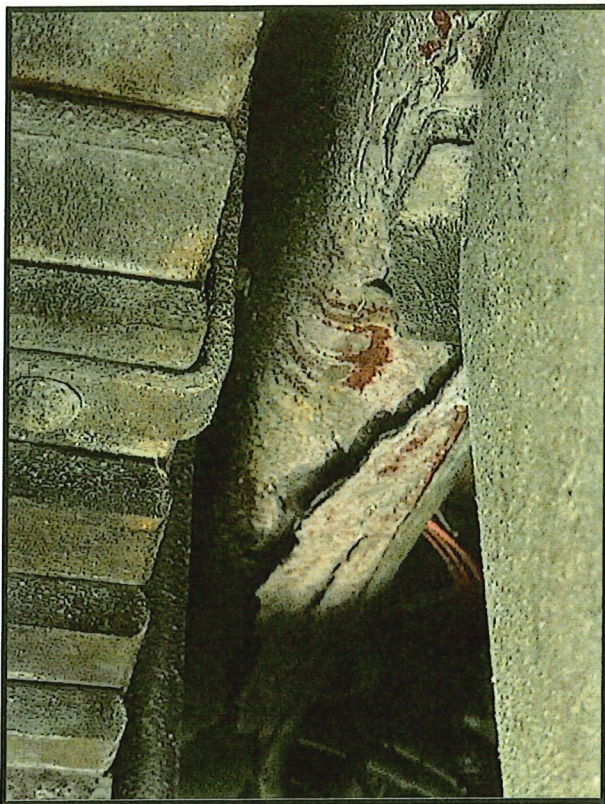
Structural Frame Rail Cracked and Delaminating
