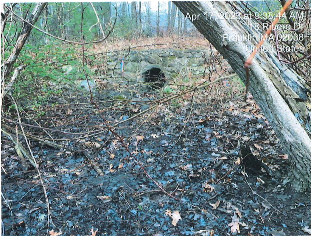
Photo 1. View of BVW origin onsite, piped from residential properties
