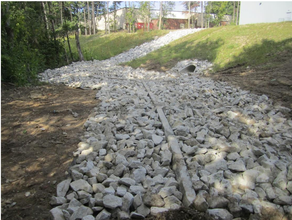
Level spreader at pond outlet
