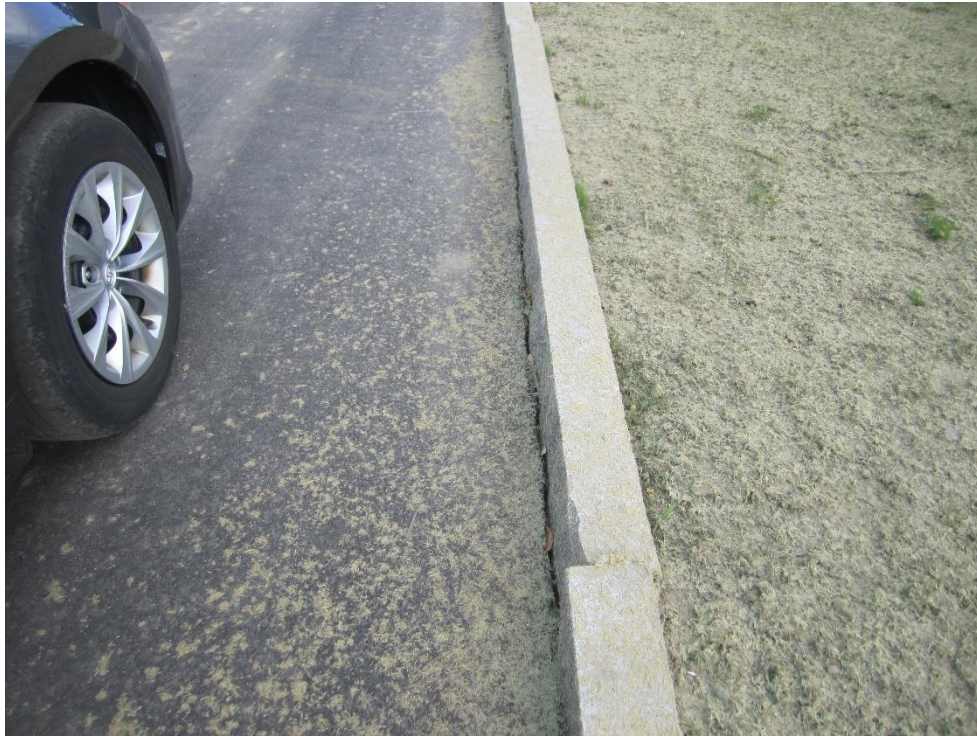
Single segment of curbing that has ½" gap remaining between pavement
