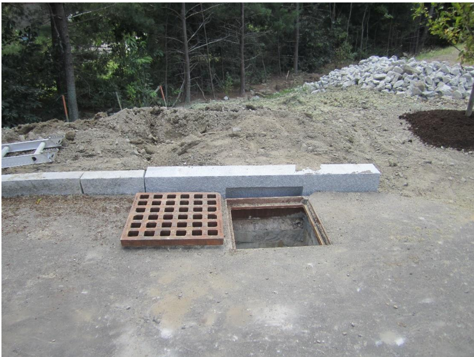
Inlet stone installed at CB-3. Contractor to add transition piece at the end.
