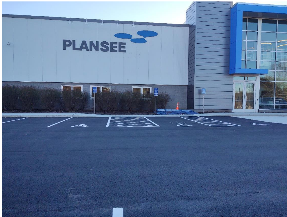
Accessible parking area. Van space lacks car stop.
