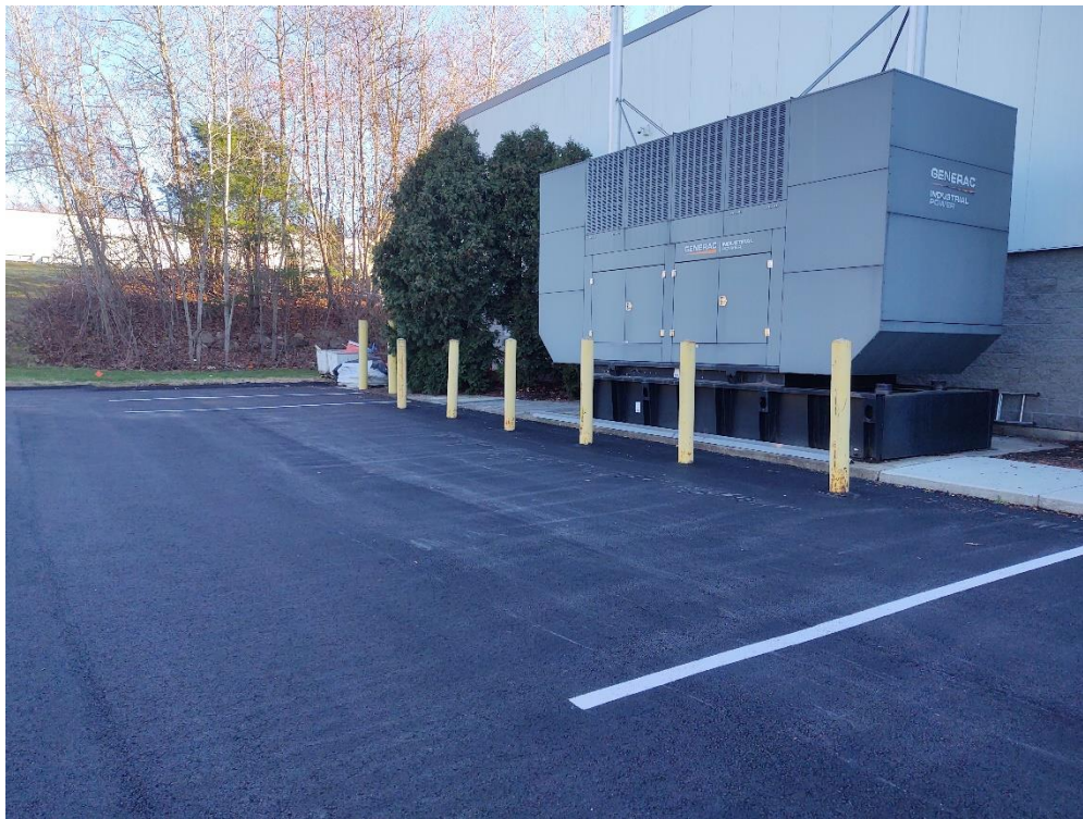
Generator pad and easterly parking spaces with bollards
