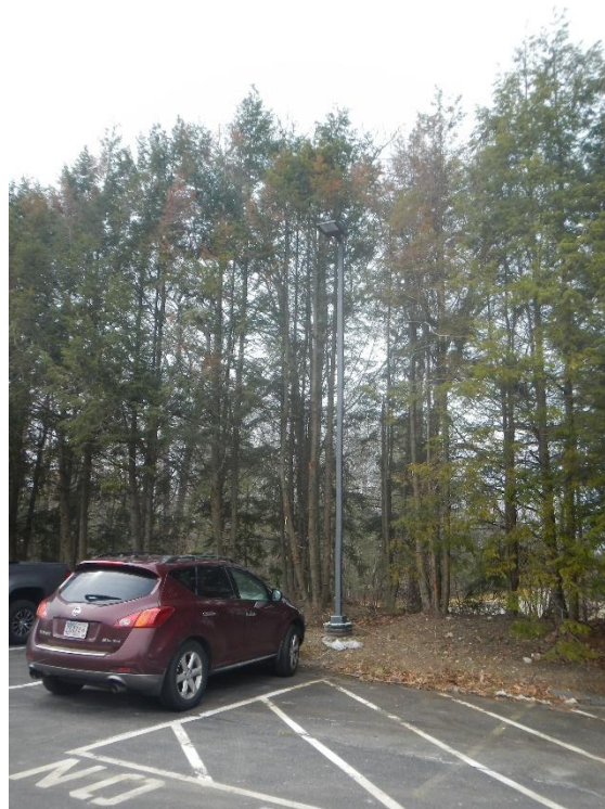
Typical light pole and luminaire installation (photo taken 3-17-23)
