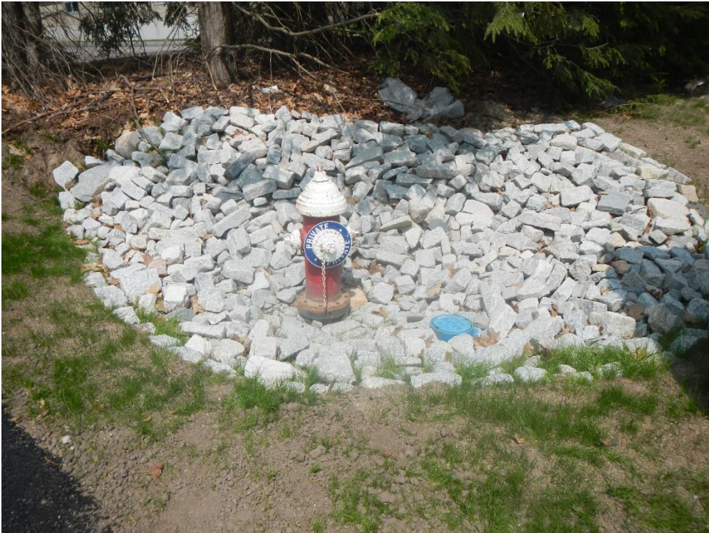
Hydrant with grading to expose breakaway flange as required (photo taken 5/9/23)
