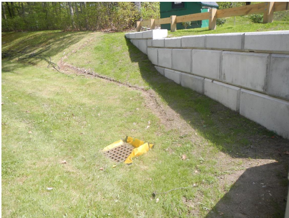
Installed block retaining wall and guardrail (photo taken 5/9/23) – silt sack has been removed
