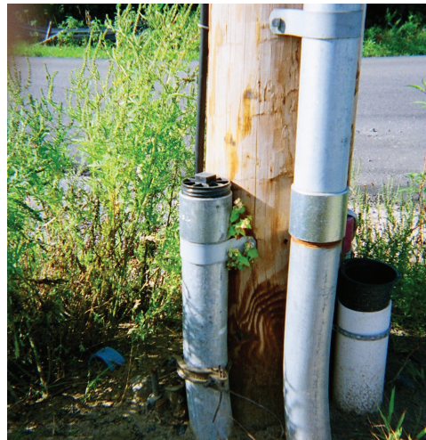
Spare Riser Sweep Spare sweep shall be bonded to down ground and capped at riser pole.
