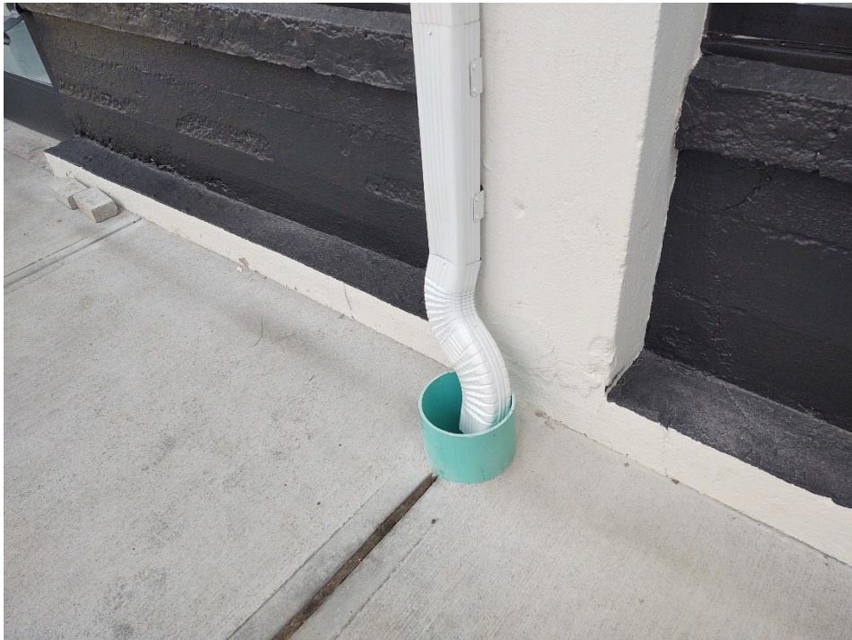
Typical downspout connection to subsurface infiltration system (photo 3/20/24)
