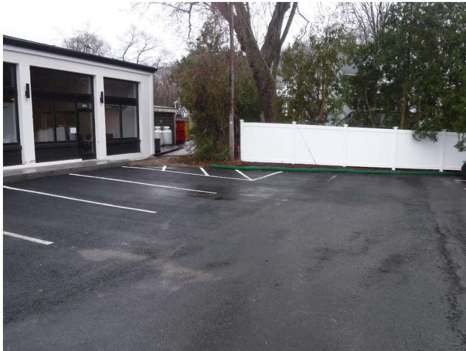
Parking adjacent to building. Hatched area where proposed accessible space eliminated.
