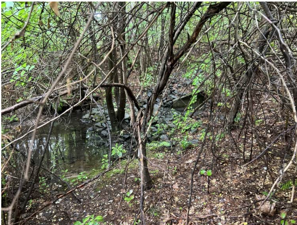
View of the rip-rap apron at the eastern extent of the channel parallel to the northern limit of work—facing north.
