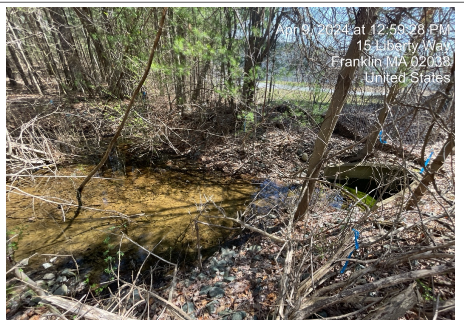
Figure 2: View of B-series stormwater IVW. Concrete flared end section visible at right.
