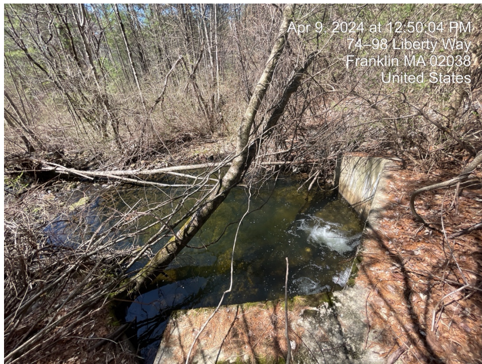
Figure 5: View of outfall from offsite detention pond. Location shown on Figure 3 above.
