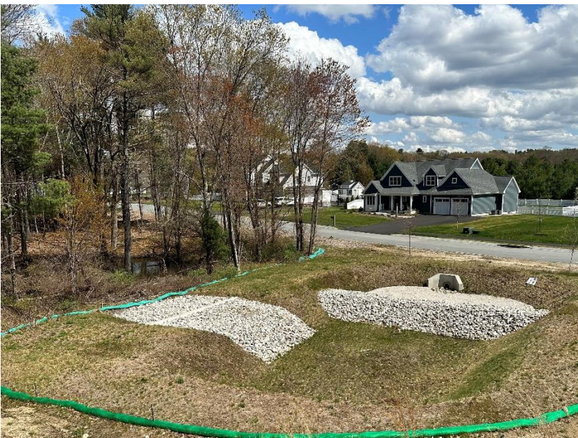
Photo 3: Completed stormwater basin along Margaret's Cove, facing east from atop the stockpile. Basin is stabilized and stockpile is bordered by erosion control tubing.
