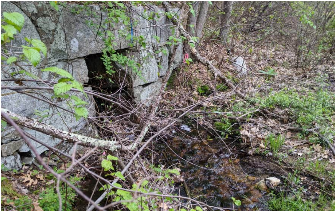
View of the unnamed tributary to Mine Brook flowing through a culvert under the Southern New England Trunkline Trail—facing northeast.
