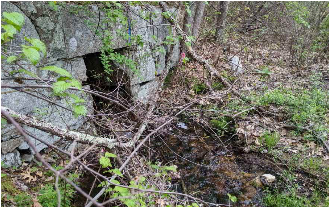
View of the unnamed tributary to Mine Brook flowing through a culvert under the Southern New England Trunkline Trail—facing northeast.
