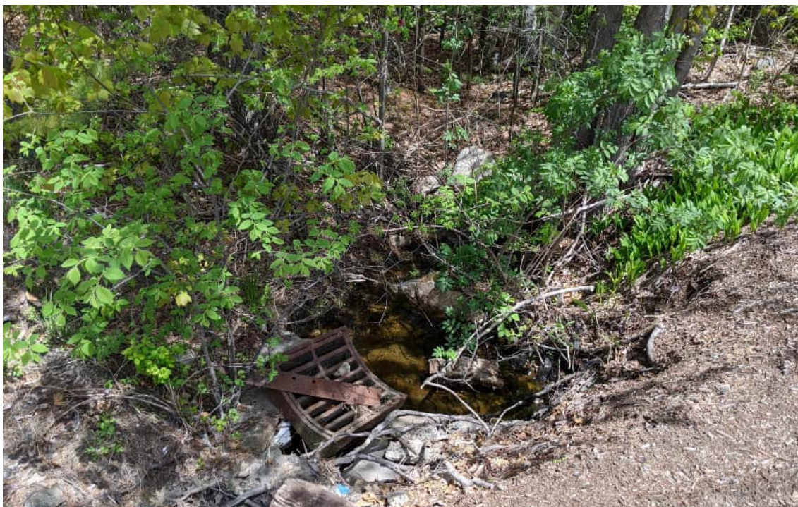
View of the unnamed perennial stream connecting the WF8 and WF9 Series BVWs at the east side of Grove Street; note the damaged infrastructure—facing east.
