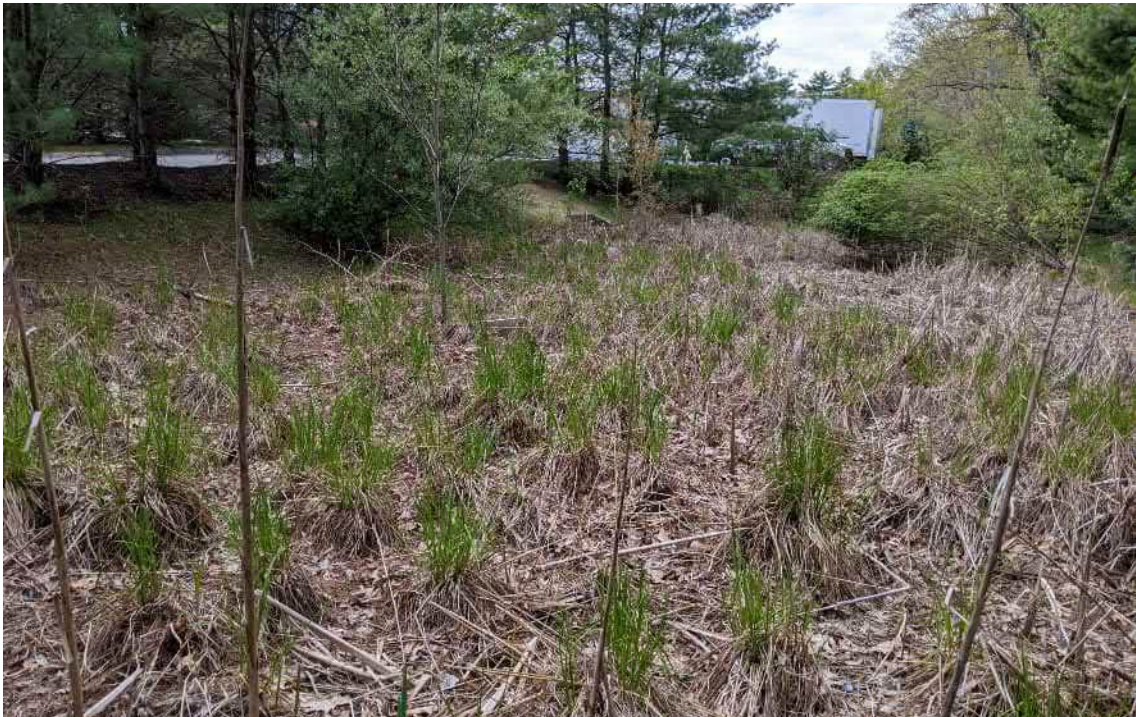
View of an unmaintained stormwater basin (WF11 Series IVW) at the northern end of the Site (157/161 Grove Street)—facing west.
