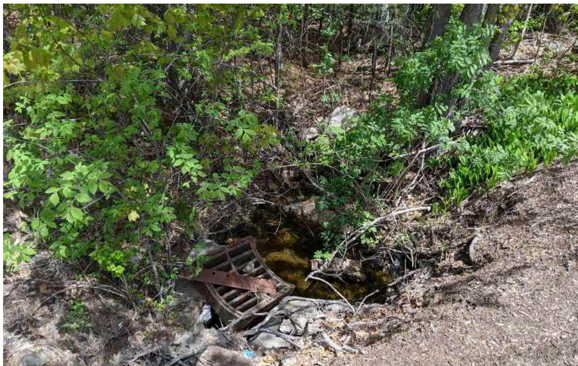
View of the unnamed perennial stream connecting the WF8 and WF9 Series BVWs at the east side of Grove Street; note the damaged infrastructure—facing east.
