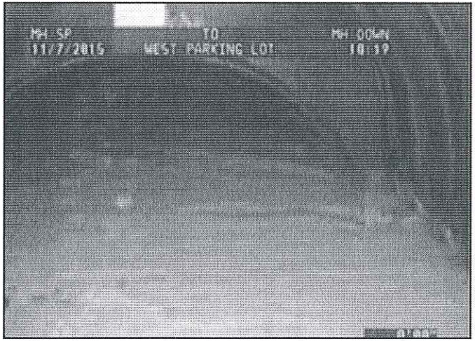
SEPARATOR ROW: Separator Row prior to cleaning
