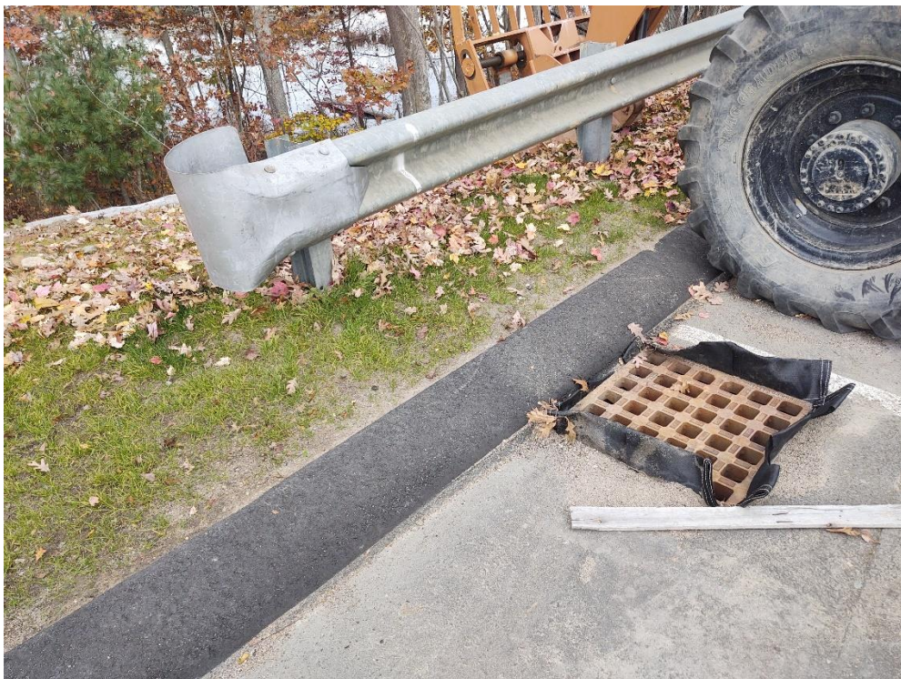
Typical installation of silt sack in catch basin
