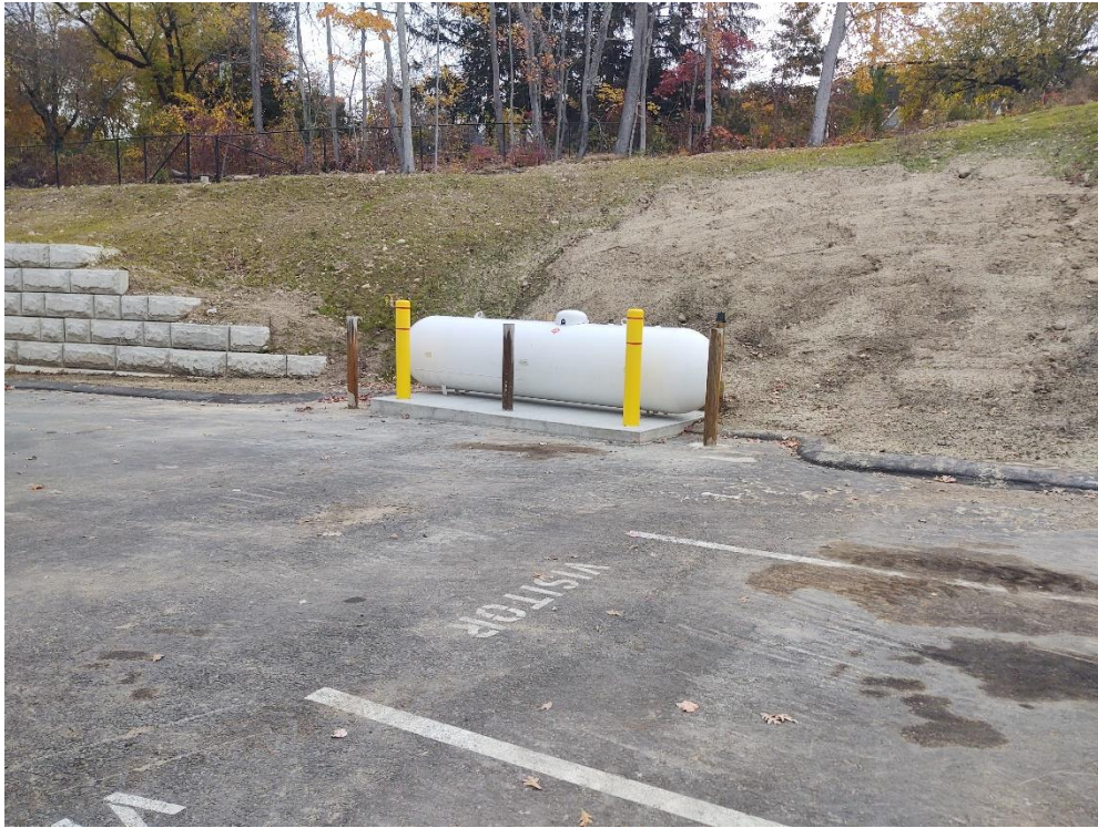
Propane tank storage area
