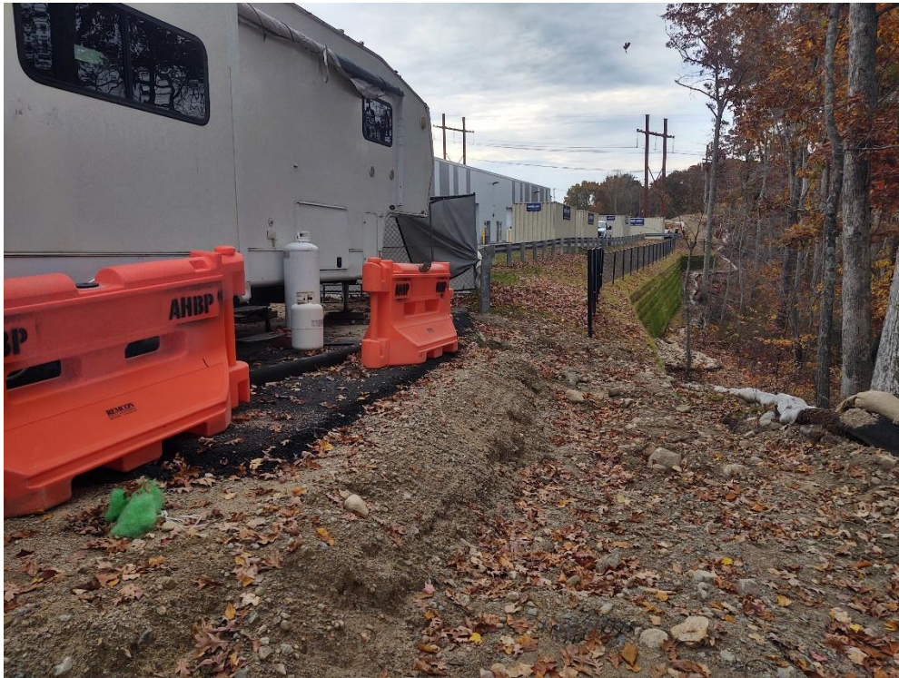
Typical temporary barrier that can be installed for slope protection, where required.
