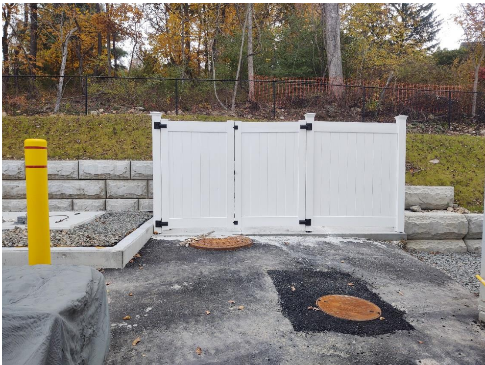
Dumpster enclosure located to the right of transformer pad
