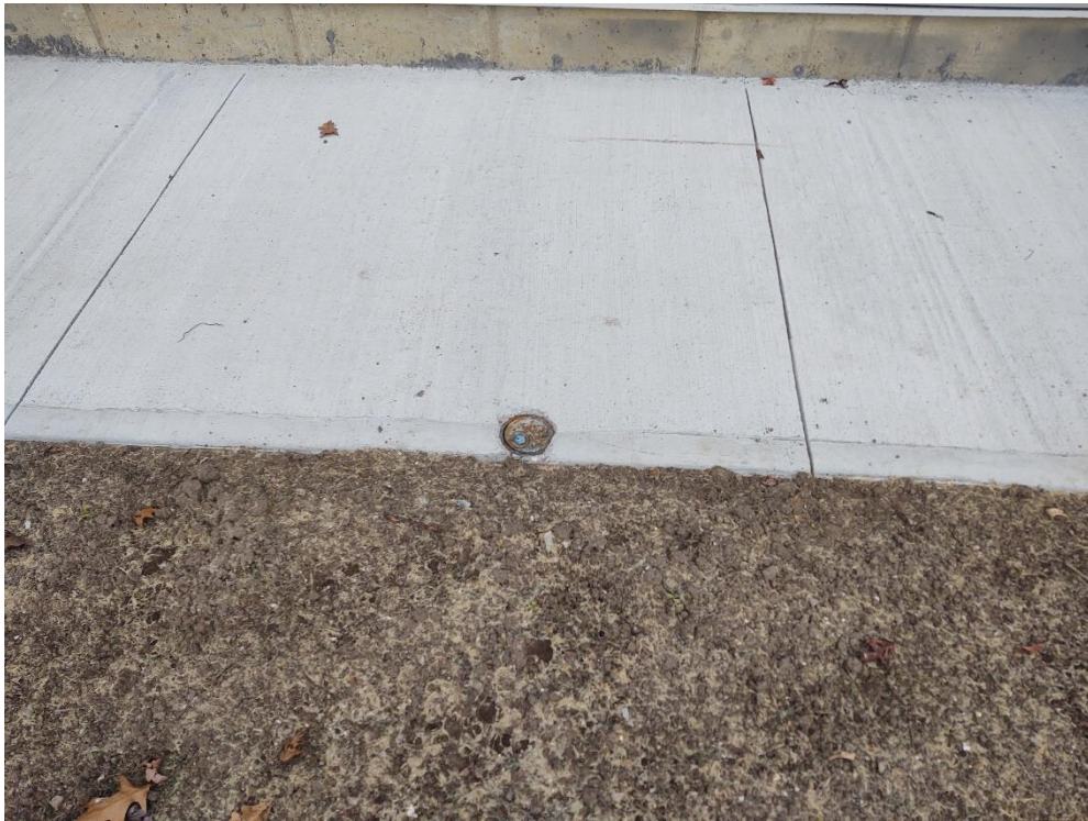
Water curb stop within sidewalk
