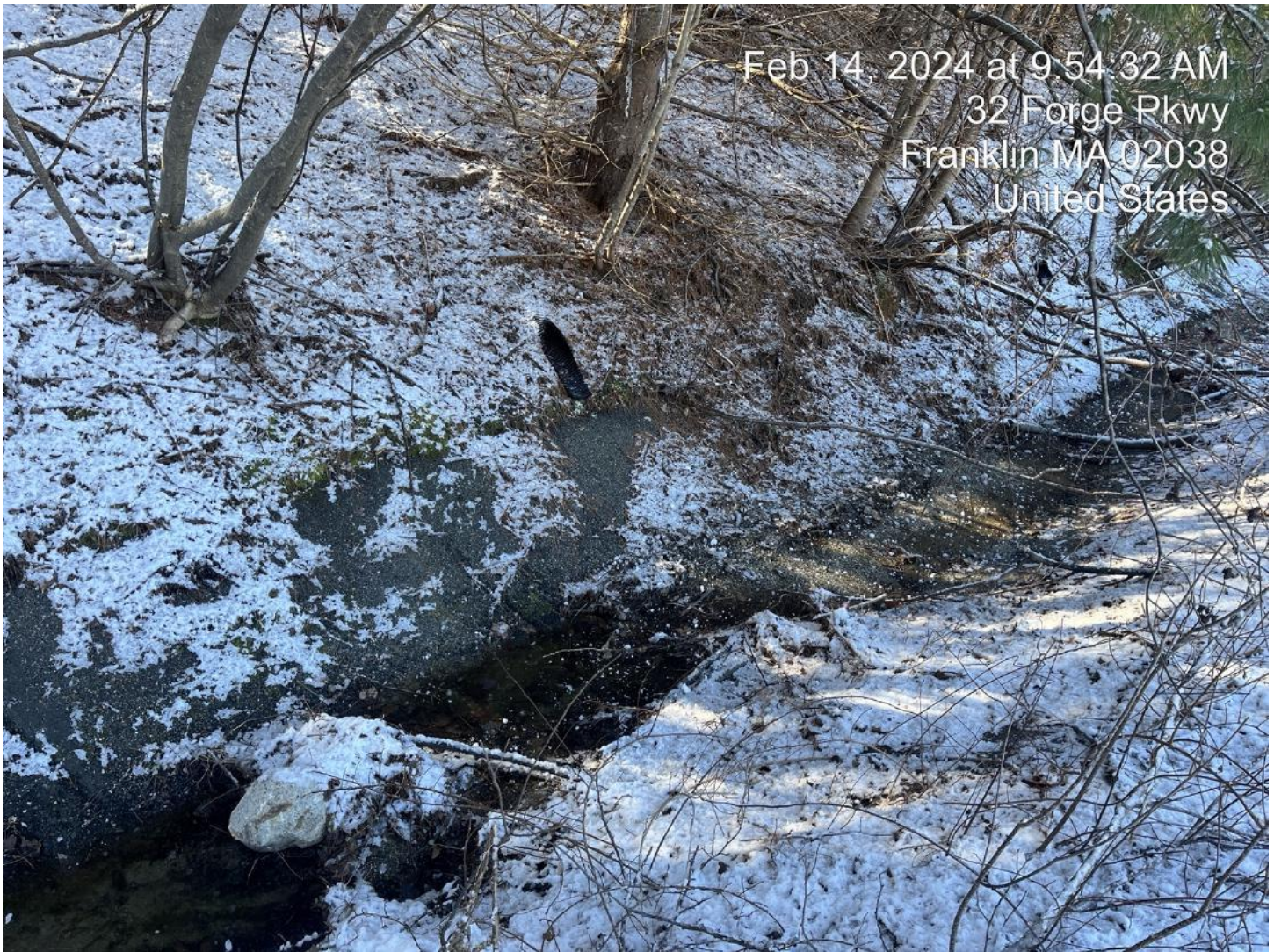
Figure 4: Additional portion of concrete drainage swale adjacent to generator pads. Drainage outlet is visible.
