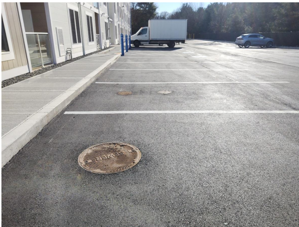
Drainage cover with "SEWER" marked
