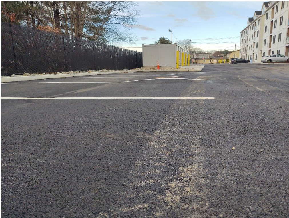
Area of pavement with raised hump
