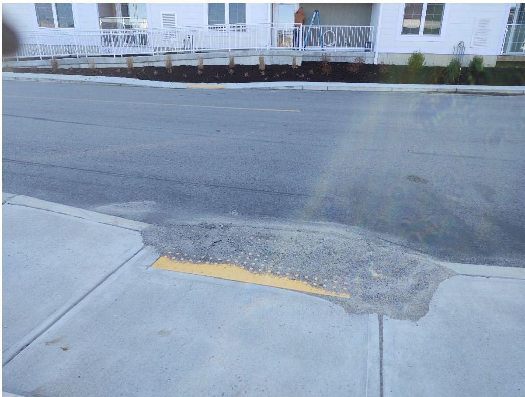
Sedimentation on ramp near Building C, possibly indicating water collection and potential icing issue
