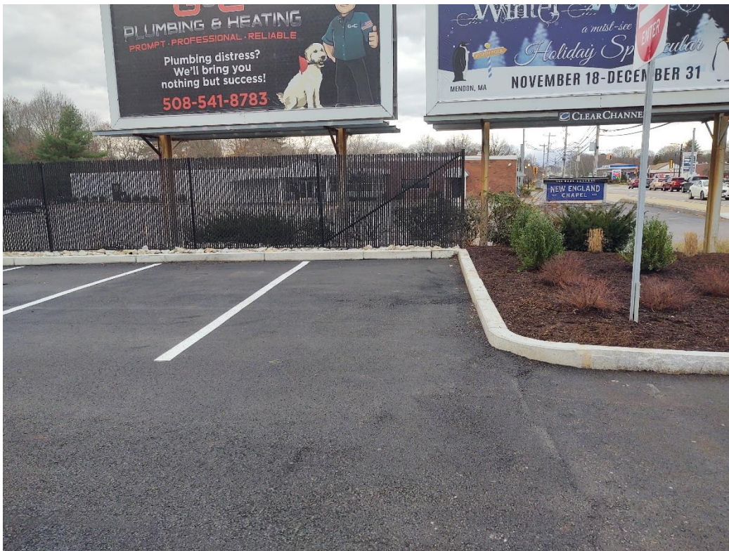
Traffic turnaround space lacking striping (right parking space)
