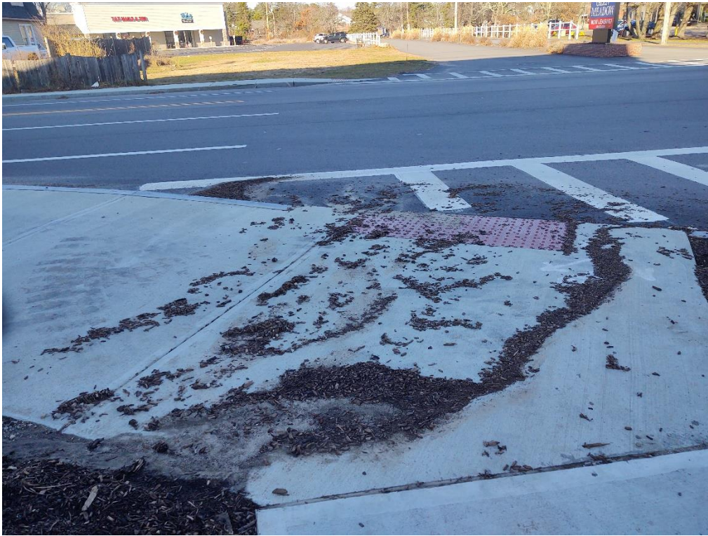
Washout onto sidewalk. No area drain installed.
