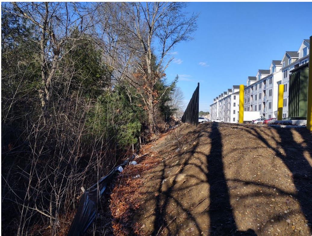
Transformer pad slope that is recommended to have rip rap installed for stabilization
