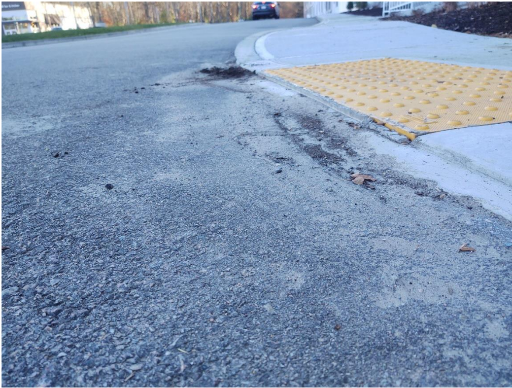
Ramp with grade transition that is anticipated to exceed ADA maximum
