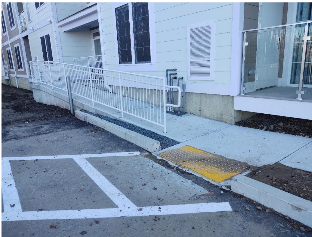
Curb ramp lacking transition curbs
