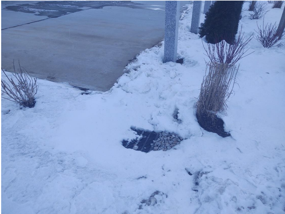
Area drain installed adjacent to patio
