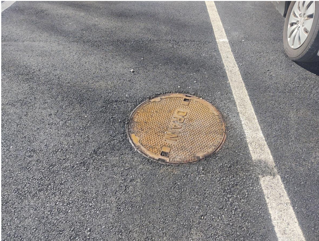
"SEWER" cover replaced with proper "DRAIN" cover
