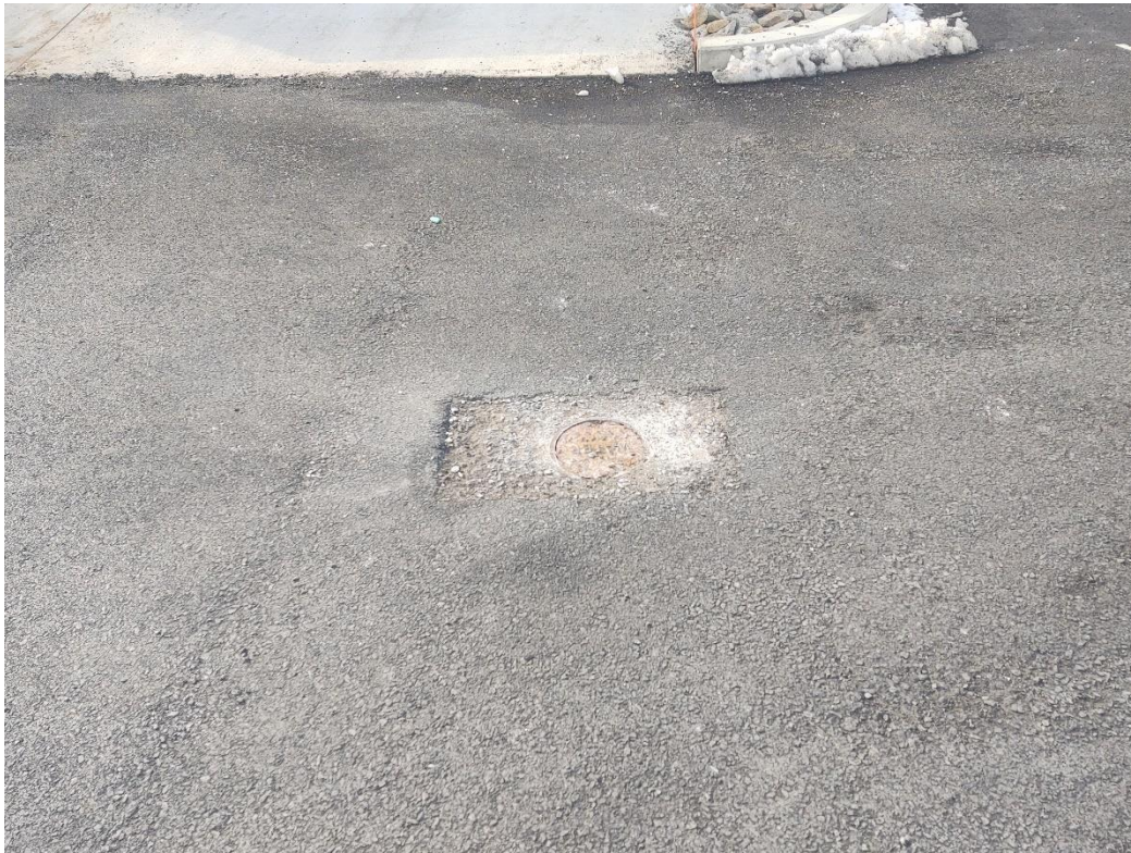
Recently installed water valve box
