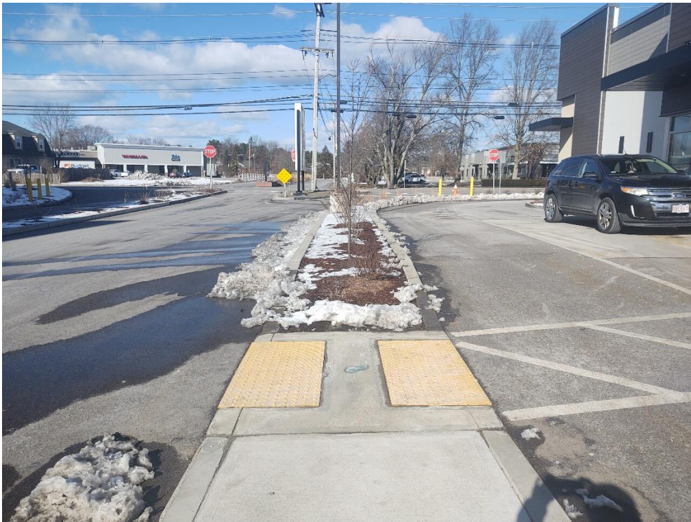
Area with additional detectable to site driveway that lacks pedestrian path
