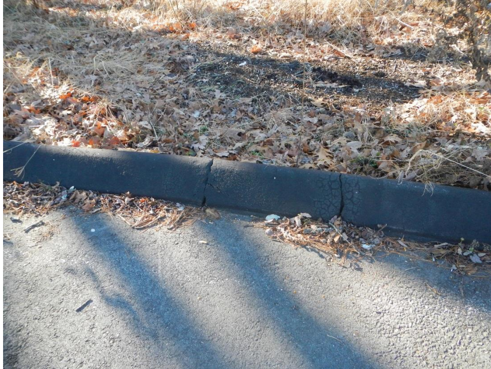
Typical bituminous curbing with minor damage
