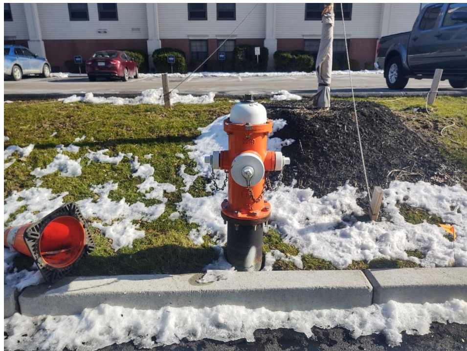
Installed fire hydrant
