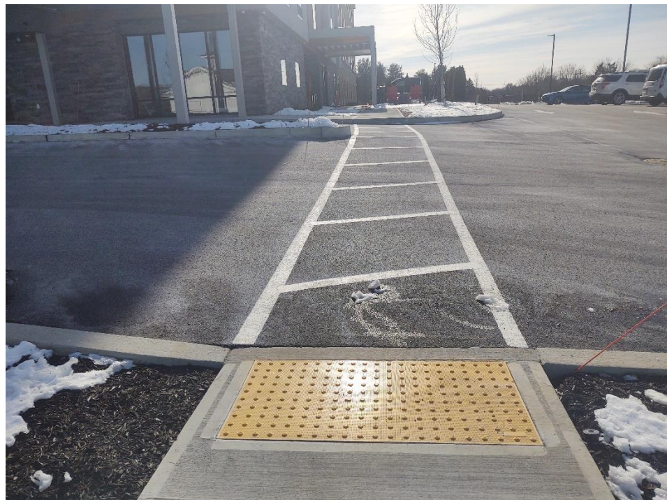
Crosswalk lacking ramp on far side
