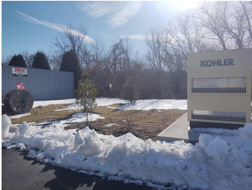
Plantings adjacent to generator pad
