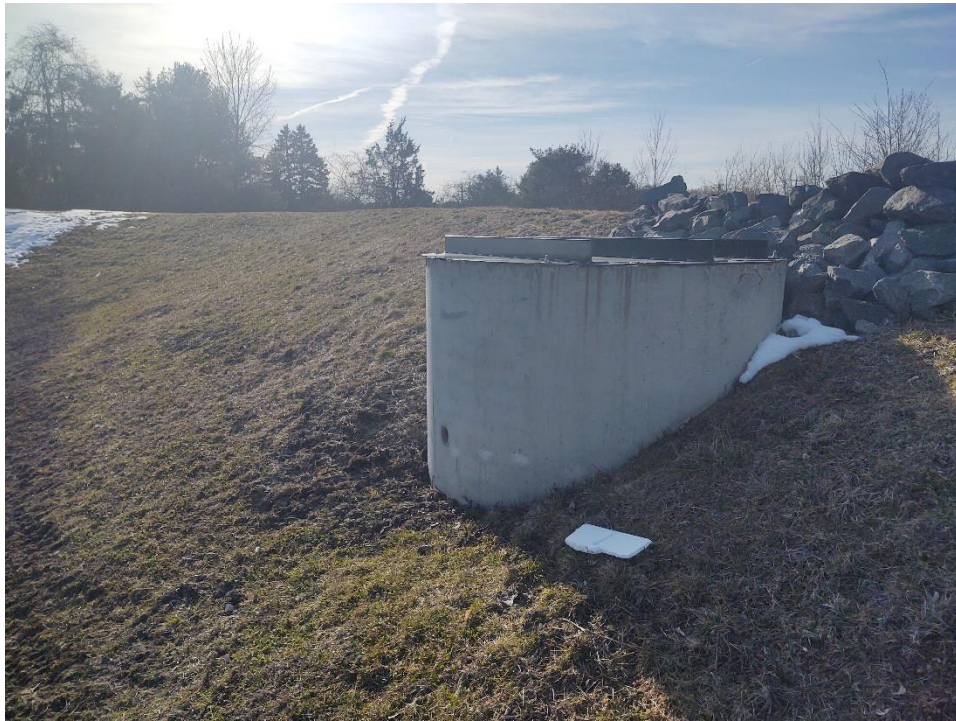
Outlet control structure
