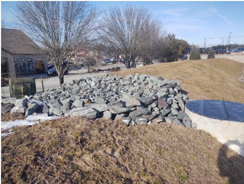
Rip rap placed higher than basin berm elevation
