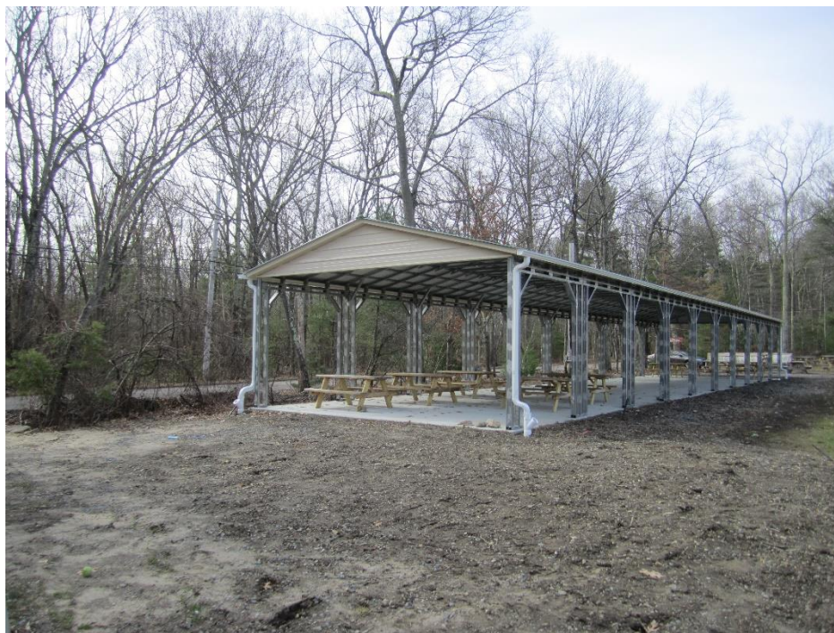
Disturbed area that is anticipated to have loam and seed installed during the grass growing season.
