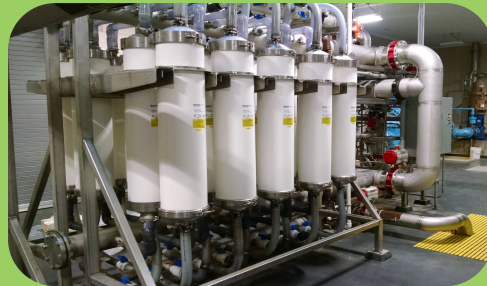
Hayward Water Treatment Plant
