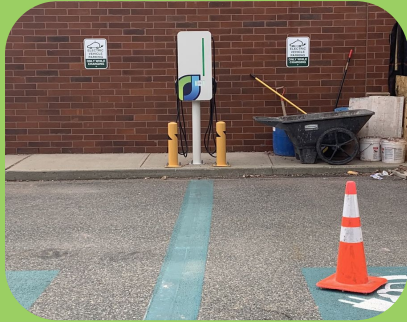
EV Charger #1 - Town Hall
