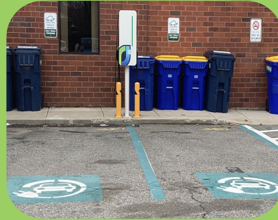
EV Charger #2 - Town Hall
