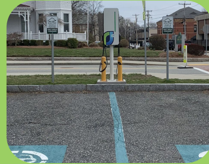
EV Charger #4 - Library
