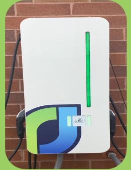
EV Charger #3 - Town Hall
