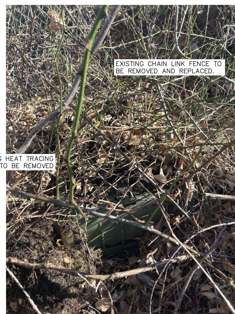
EXISTING HEAT TRACING PEDESTAL (APPROX. STA 04+25)
