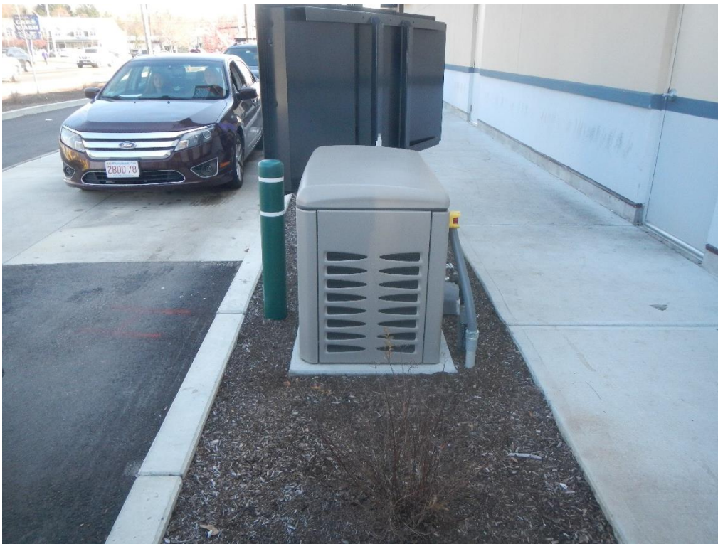
Emergency generator for sewer pump station
