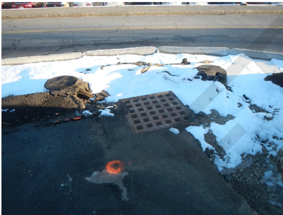
Area lacking curbing, guardrail, and fencing at southeast corner of lower parking area
