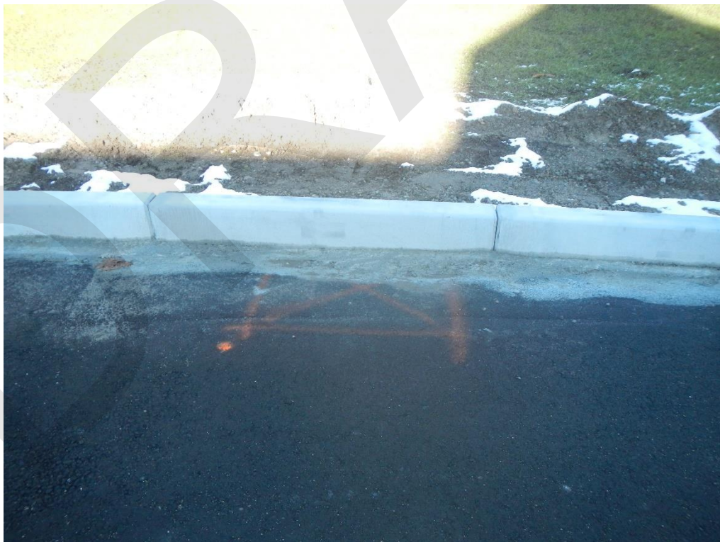
Typical catch basin currently covered by binder course
