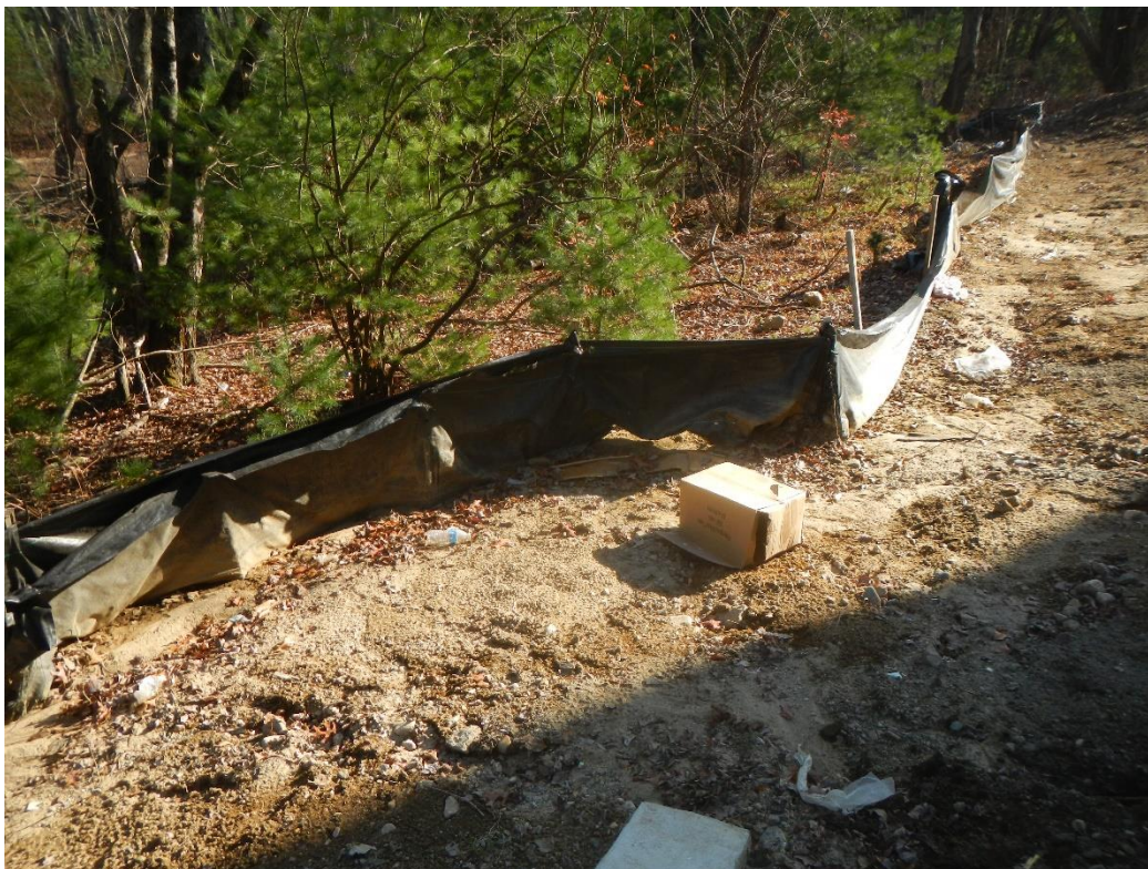
Typical break in erosion and sedimentation controls
