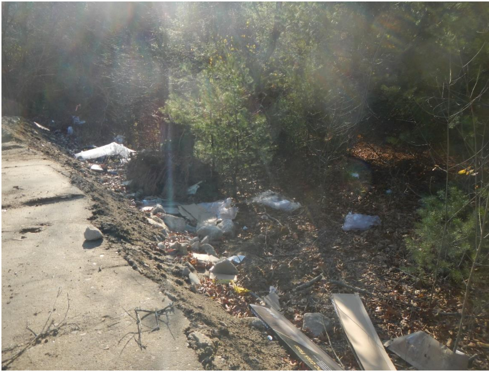
Typical trash in residential construction area that requires cleanup
