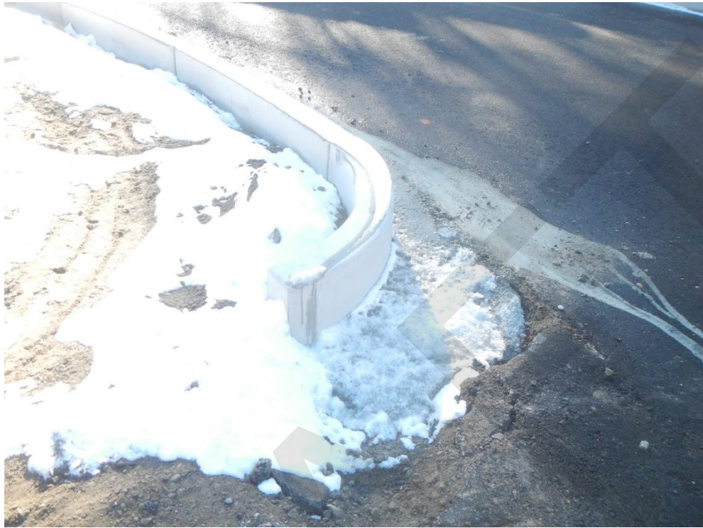
Concrete curb that lacks transition curb
