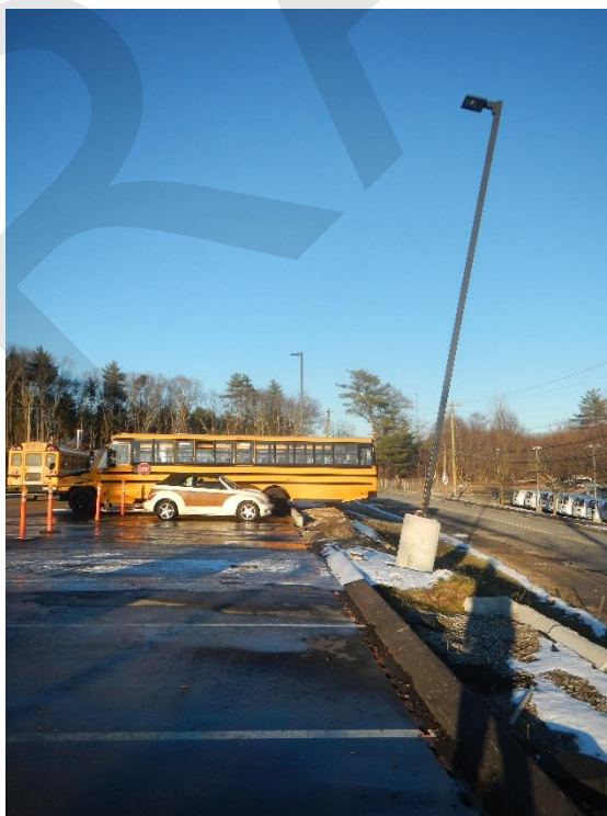
Damaged pole and foundation in lower parking area
