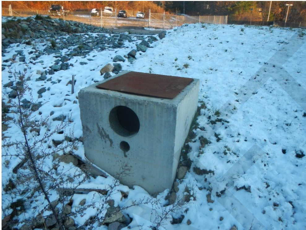
Outlet control structure that lack grate
