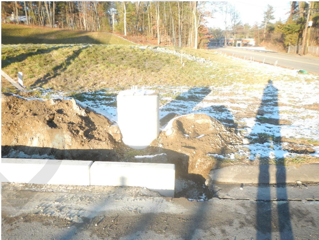
Incomplete lighting and curbing at site entrance
