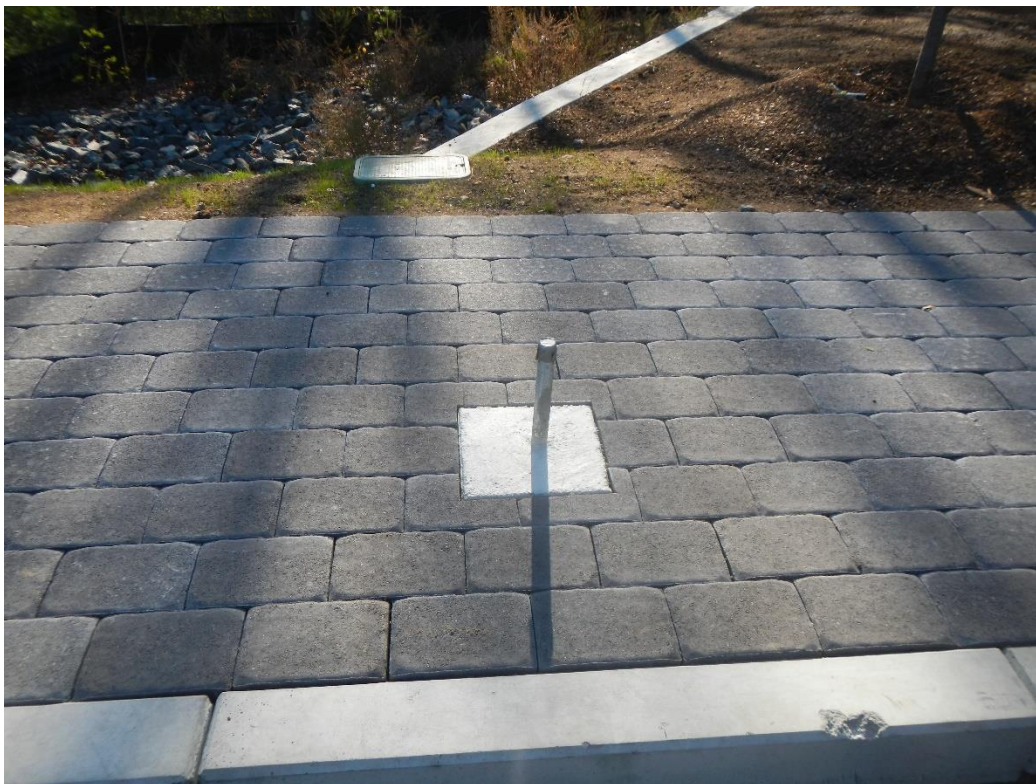
Conduit for electric vehicle parking station
