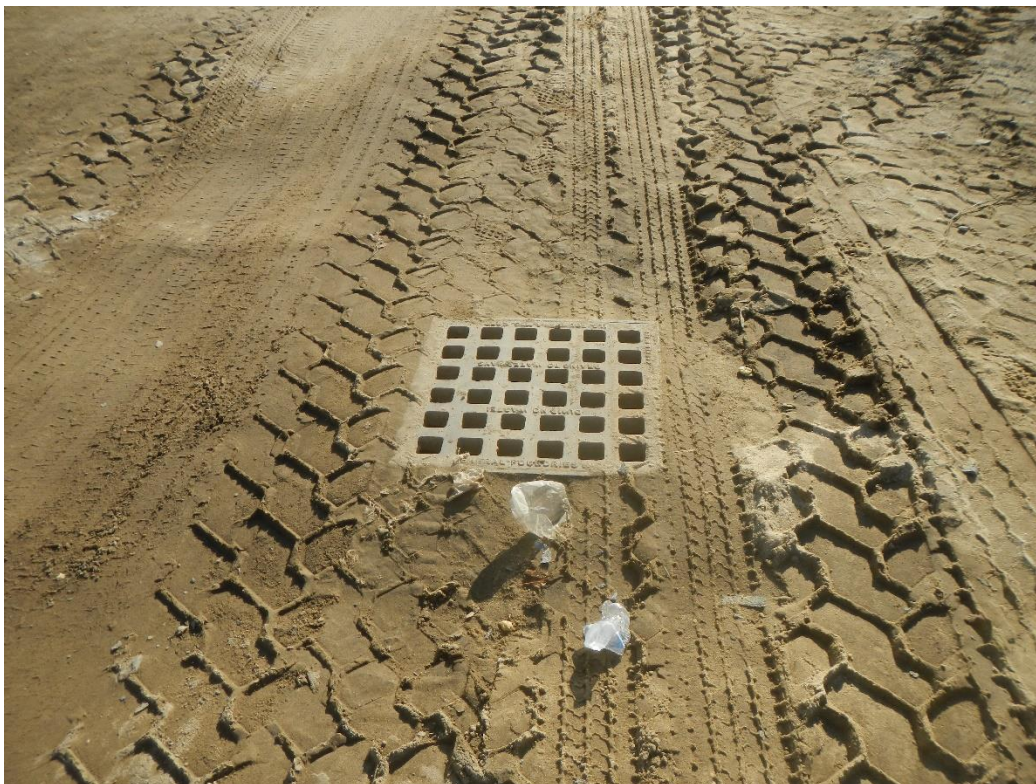
Catch basin lacking silt sack in residential construction area
