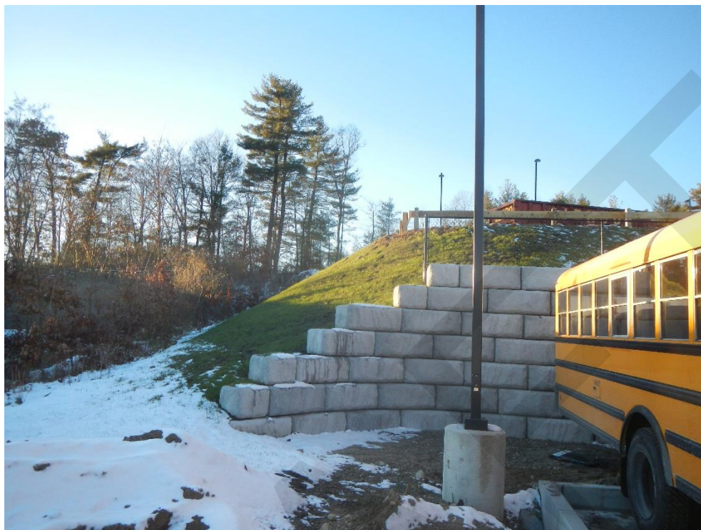
Portion of Retaining Wall No. 2 that may require additional fencing for fall protection
