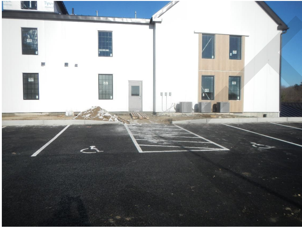
Accessible parking area lacking signage and route to building
