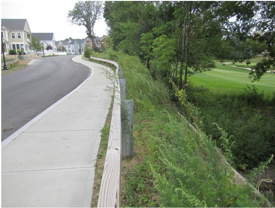
Retaining wall lacking fencing
