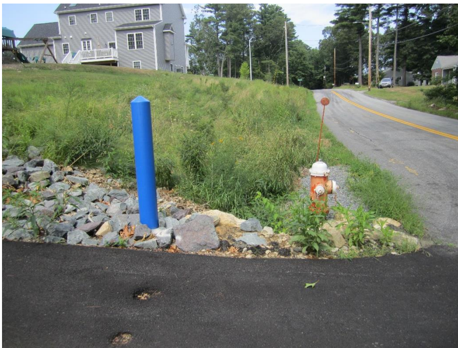
Bollard installed adjacent to driveway to protect hydrant (not part of subdivision)
