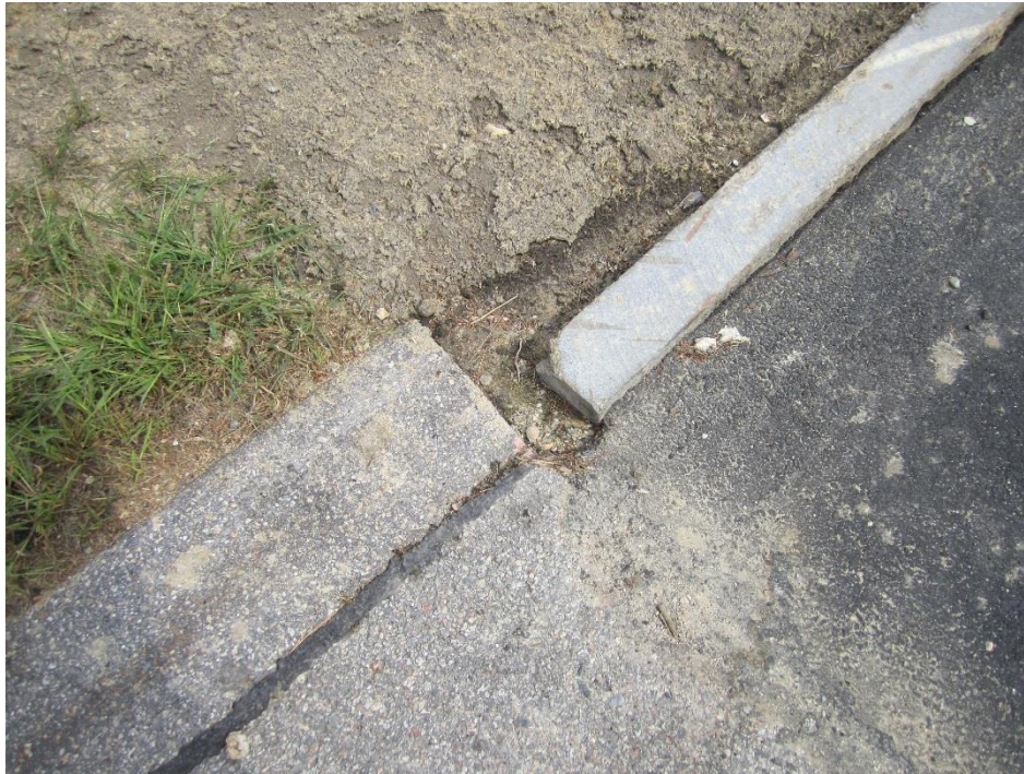
Gap between curbing at Brandywine Road
