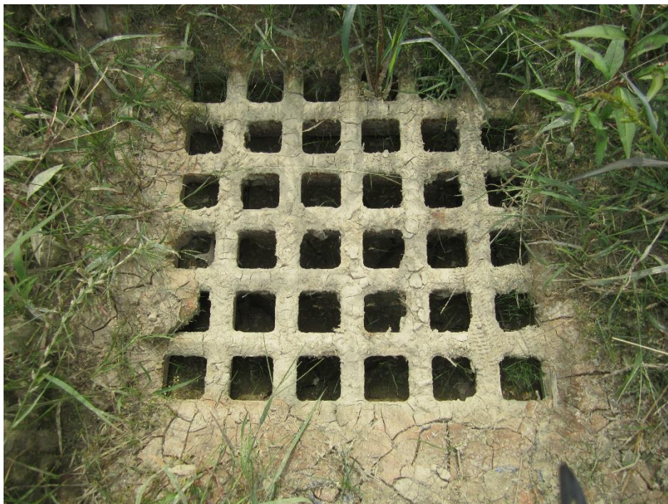
Catch basin that requires removal of filter fabric and possible cleaning
