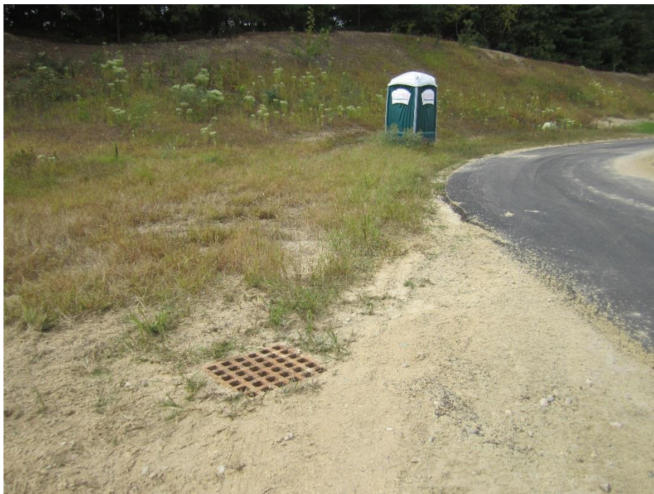
Swale that requires regrading plus loam and seed near cul-de-sac
