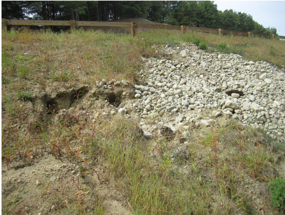
Erosion on slope located above retaining wall
