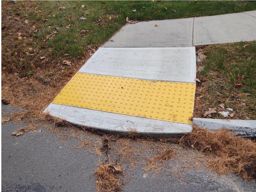
Ramp located not flush with pavement at Prospect Street
