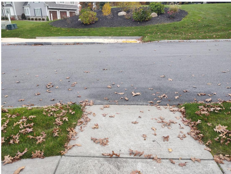
Accessible ramp lacking detectable warning panel
