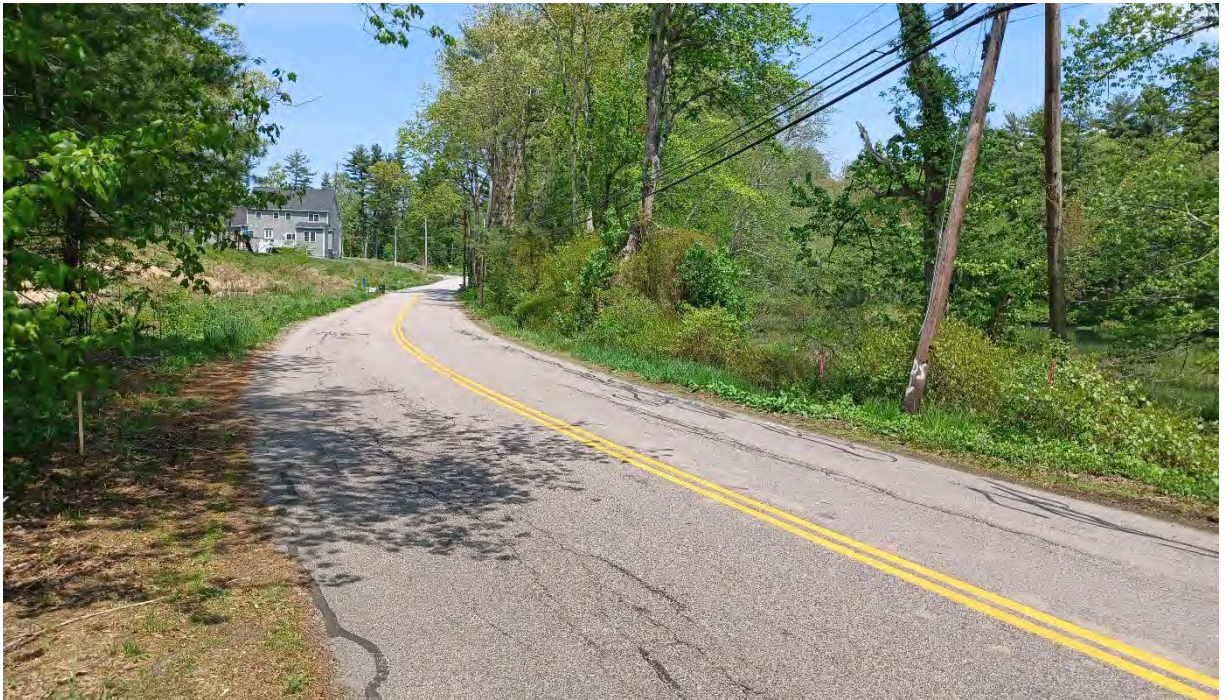
Photo #4: View of existing P49 and stake for new stub pole P49-90. A guy will extend from P49 to P49-90 to support the removal of the existing push brace. Facing north.
