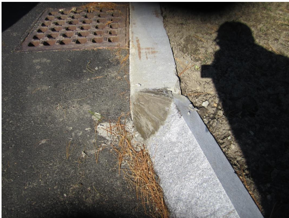
Concrete placed at interface between slant granite curb and drainage inlet stone
