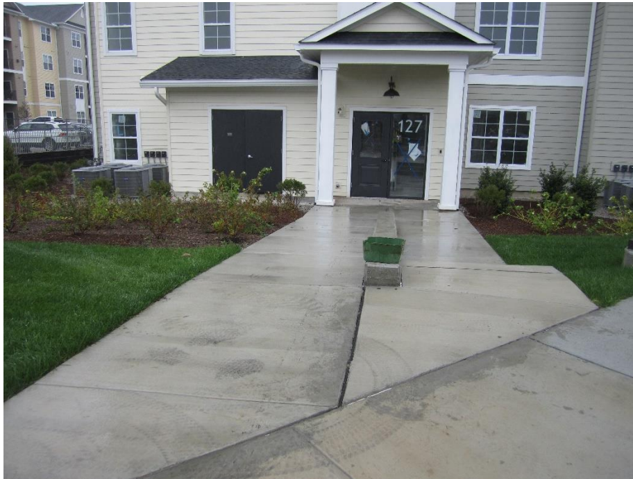
Building entrance lacking handrails
