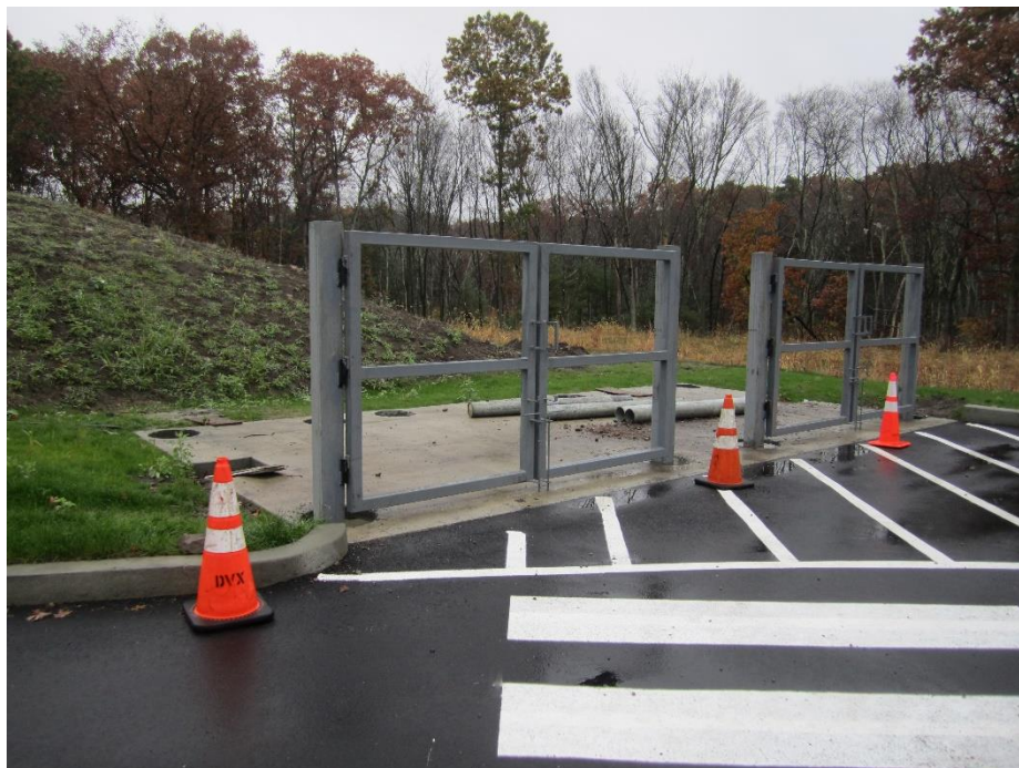
Incomplete dumpster enclosure
