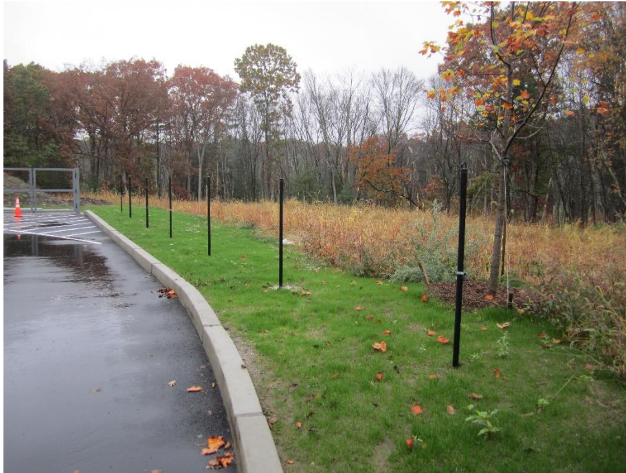
Chain link fence has not been installed
