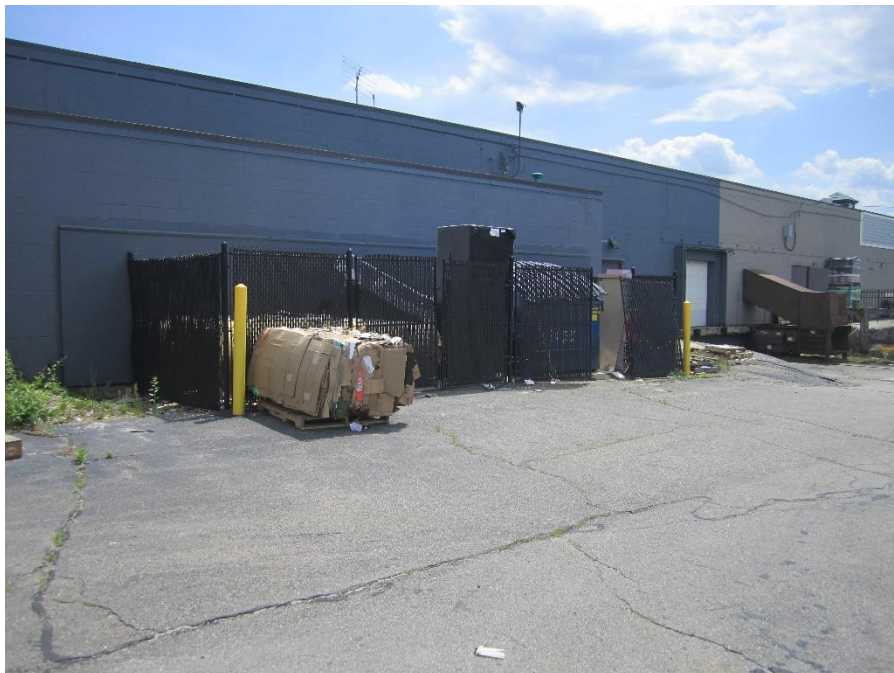
Dumpster area requiring maintenance to enclosure
