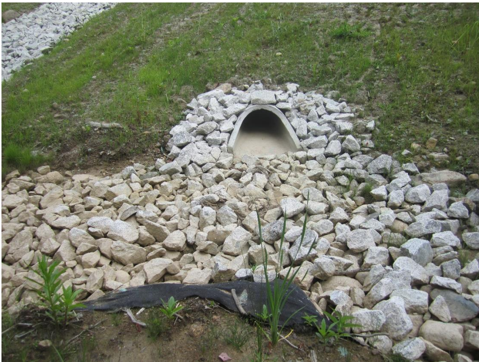
Pond outlet that lacks concrete level spreader
