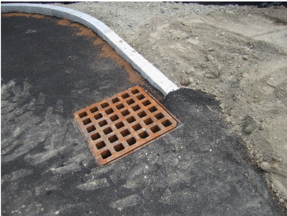
Catch basin that is recommended to have curb extended and brought flush with pavement
