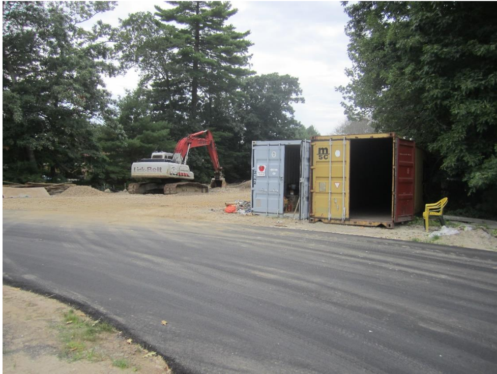
Laydown area requiring restoration
