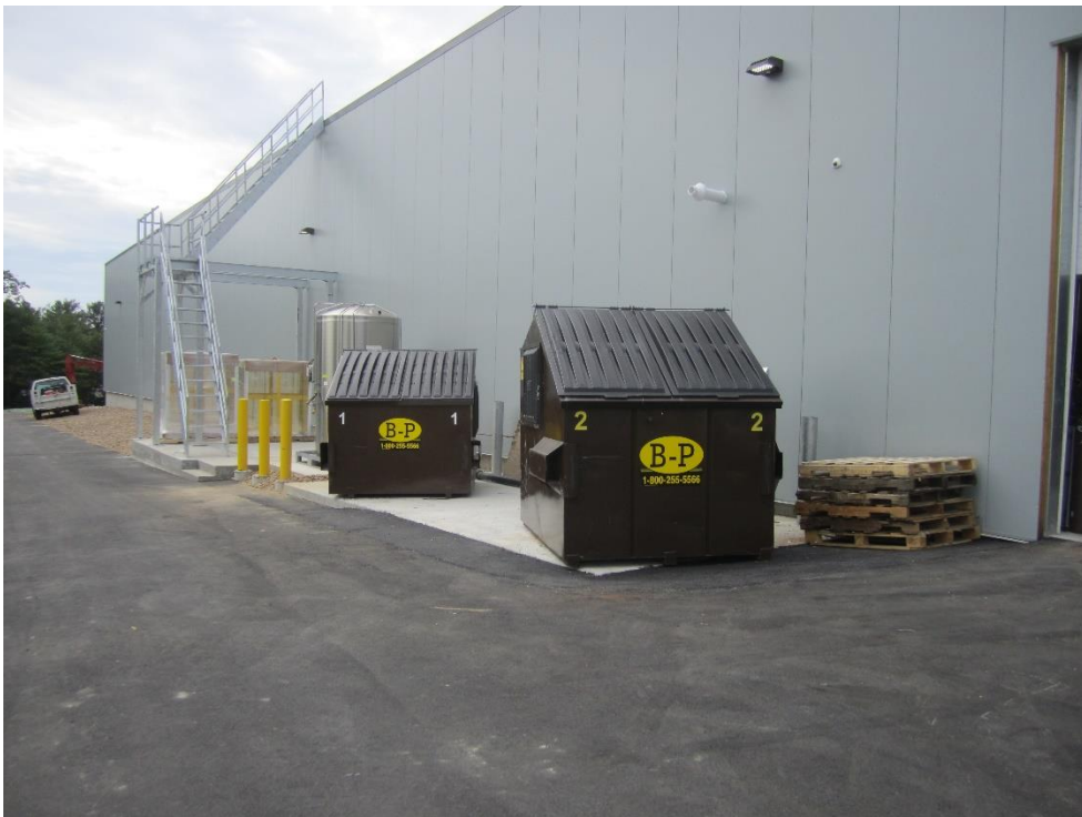
Dumpster area lacking enclosure and roof access lacking fencing
