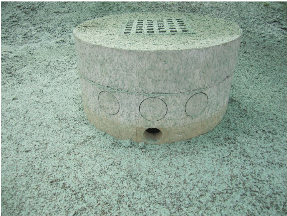
Outlet control structure that requires removal of 8" orifice knockouts
