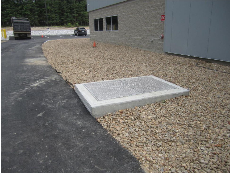
Sewer pump chamber access installed above grade per direction of Water and Sewer Superintendent.
