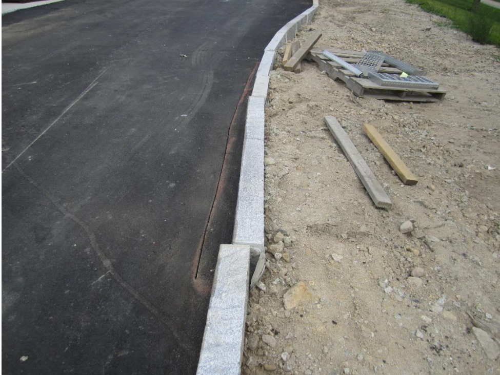
Typical curb that is required to be reset
