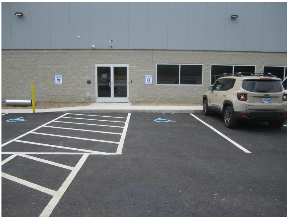
Accessible space that requires curb cut (ramp) to sidewalk
