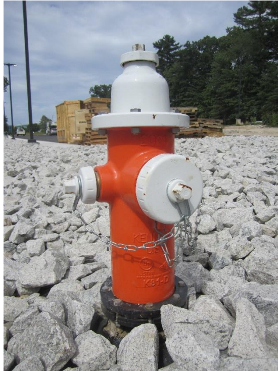
Town standard fire hydrant
