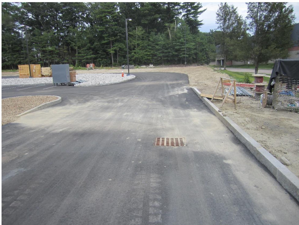
Catch basin not installed adjacent to curb (curb line shifted as part of approved field change)
