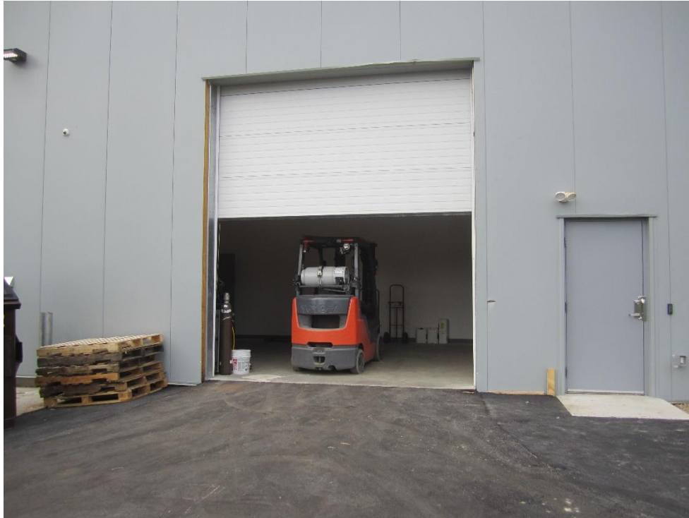
Door lacking bollards
