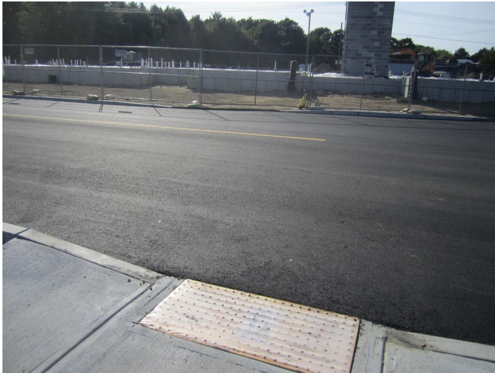
Area that BETA does not recommend installing crosswalk until Building A has been constructed.
