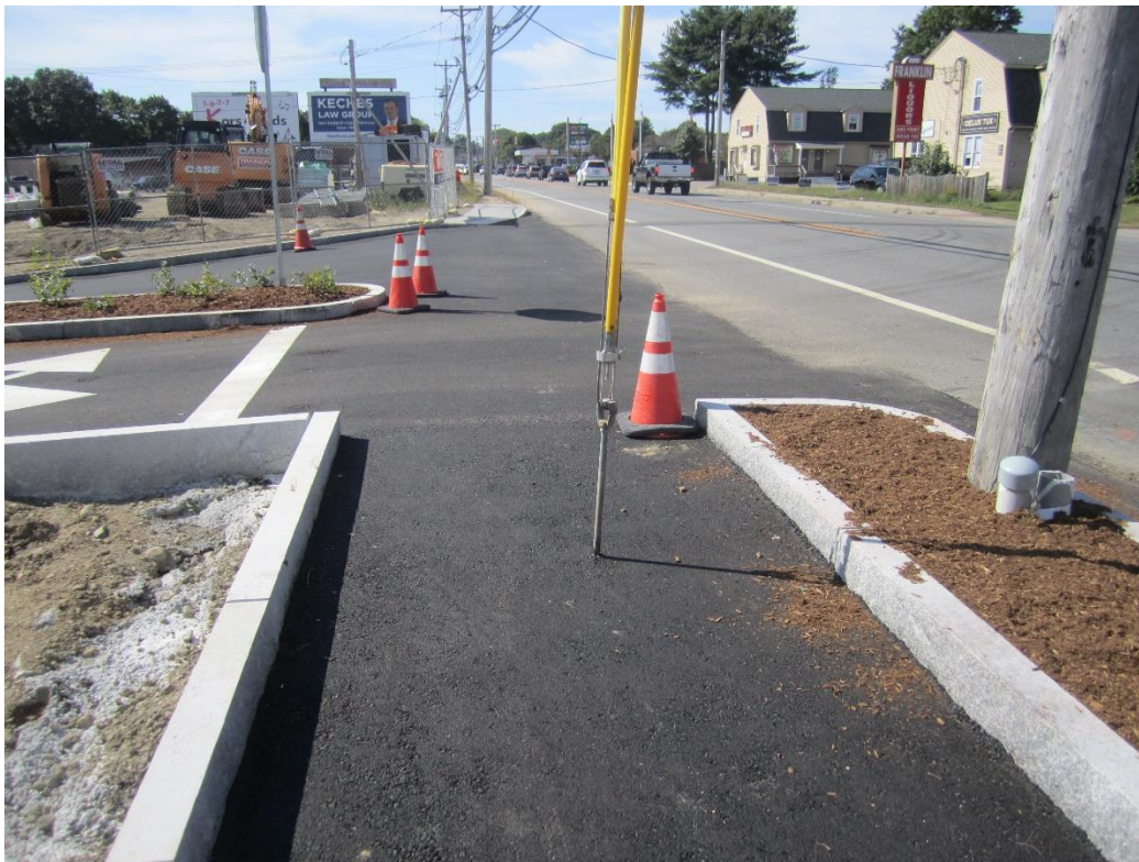
Guy wire (to be relocated) in pedestrian path along frontage of property. Crosswalk has not been striped.
