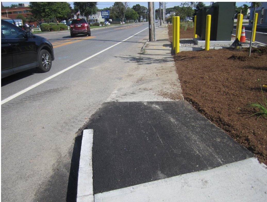
Temporary bituminous transition from ramp to existing curb cut along frontage of property.
