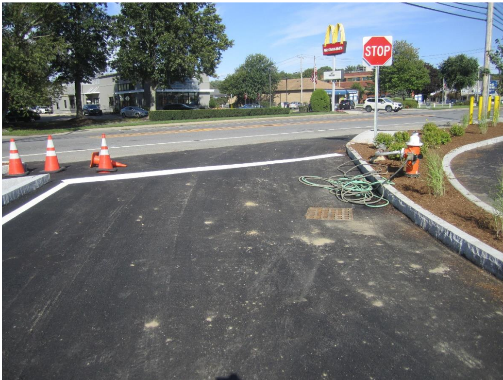
Catch basin not installed against curb line and with steep cross slope of pavement
