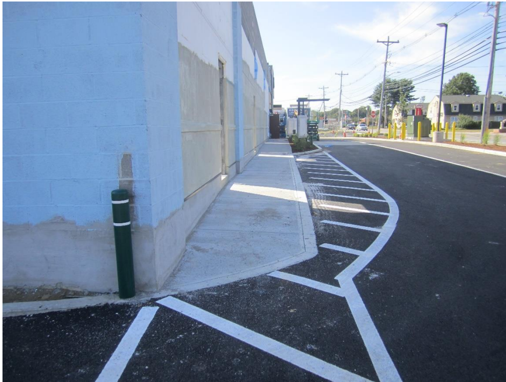
Sidewalk added to north side of Building C with ramp that lacks detectable warning.
