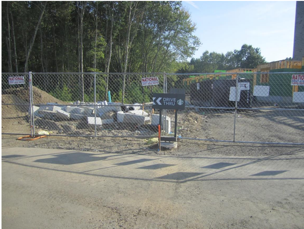
Typical drive-thru directional signage
