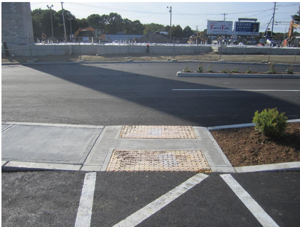
Area with additional ramp to site driveway that lacks pedestrian path.
