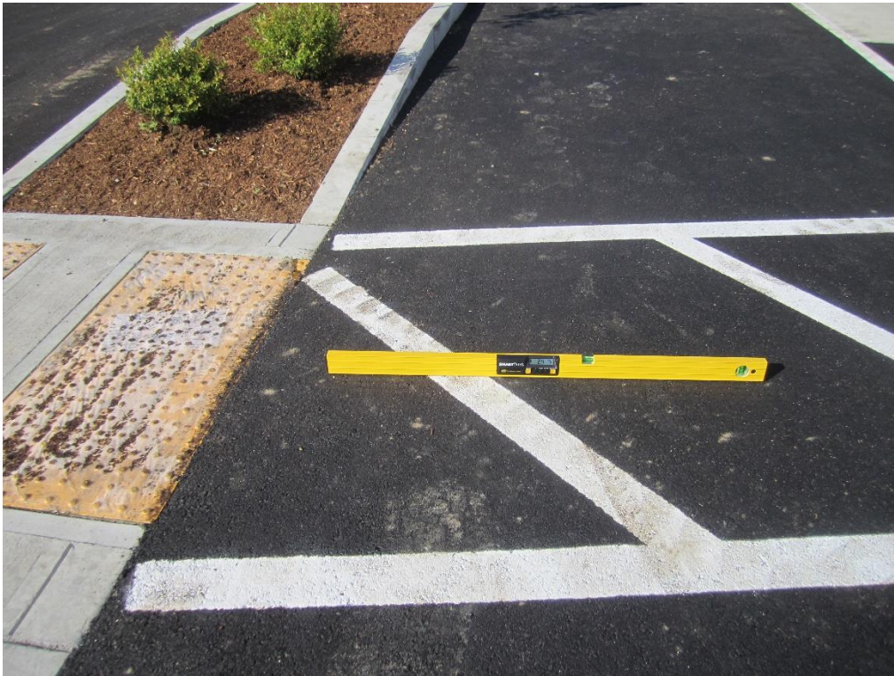
Grading may direct stormwater onto ramp
