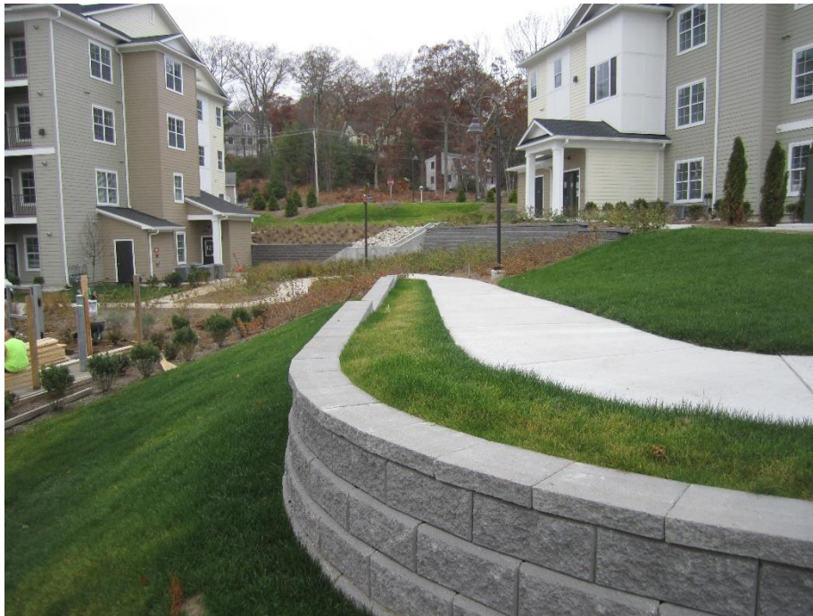
Fence has not been installed on the retaining wall between Buildings 3 and 6
