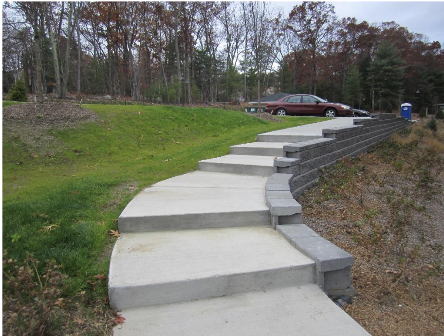
Handrails have not been installed on the stairs to the west of Building 6
