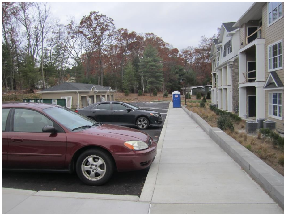
Fence has not been installed along retaining wall to the west of Building 6
