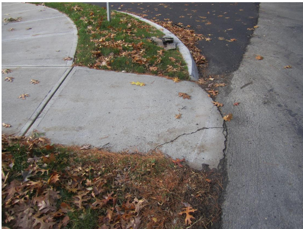
Damaged sidewalk/ramp panel at intersection of Prospect Street.
