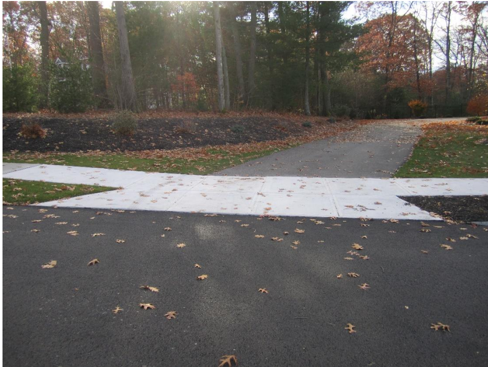
Depressed sidewalk at Lot 5. No accessibility issues noted.
