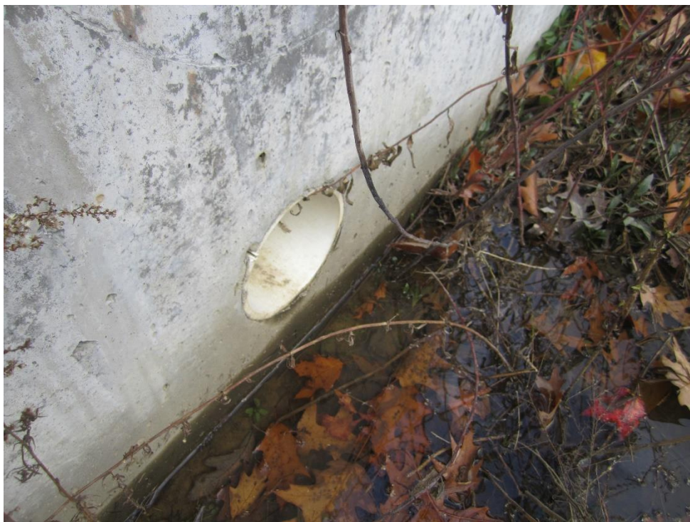
Infiltration Basin No. 1 outlet orifice that lacks cover plate
