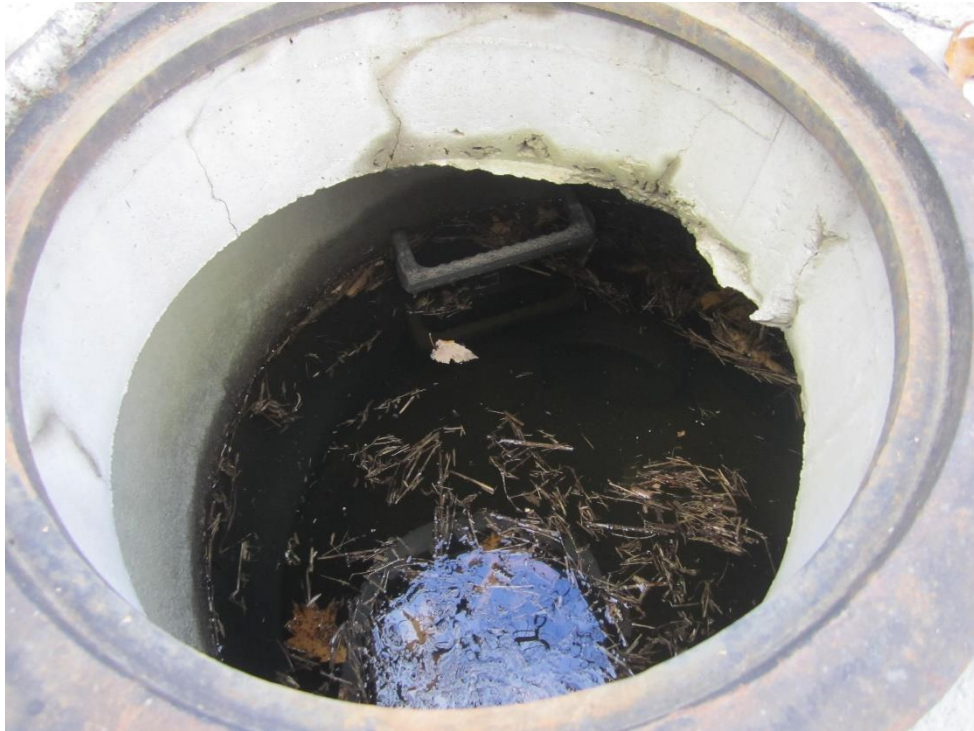
Infiltration Basin No. 2 Outlet Control Structure with grate removed (currently on ground)
