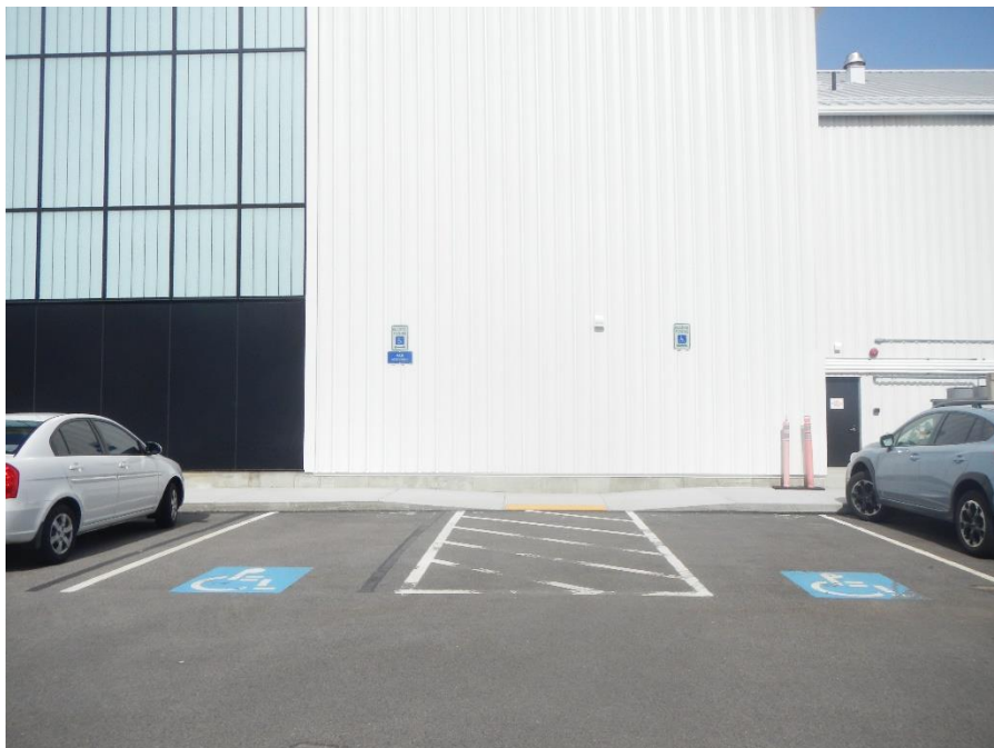
Accessible signage, possibly mounted higher than permitted
