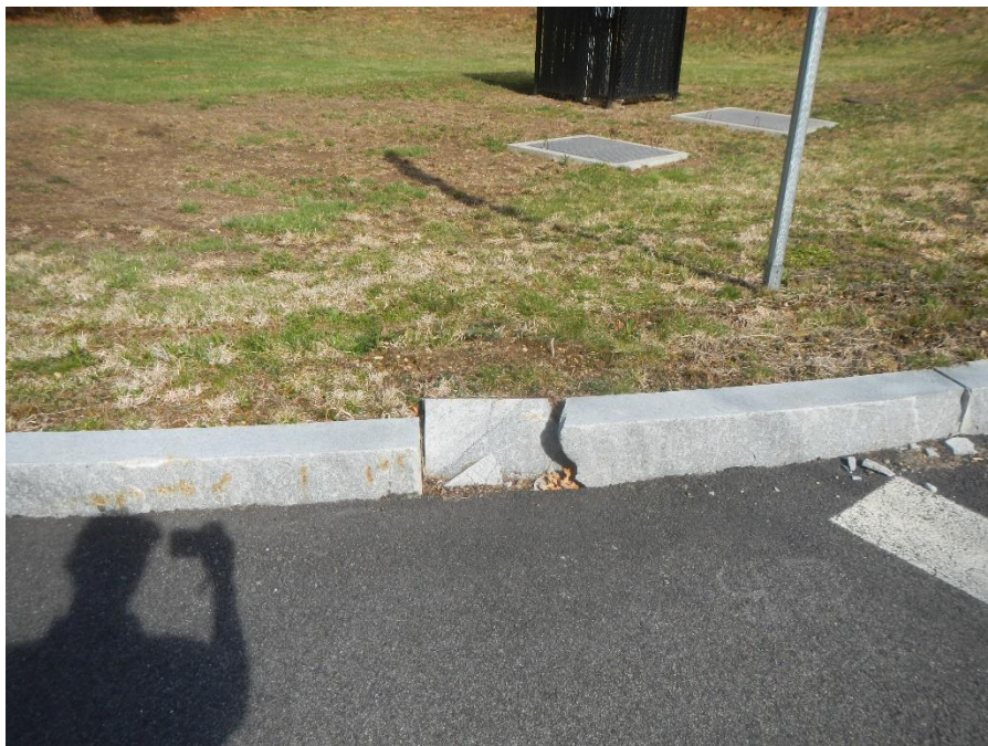
Damaged curb at site exit
