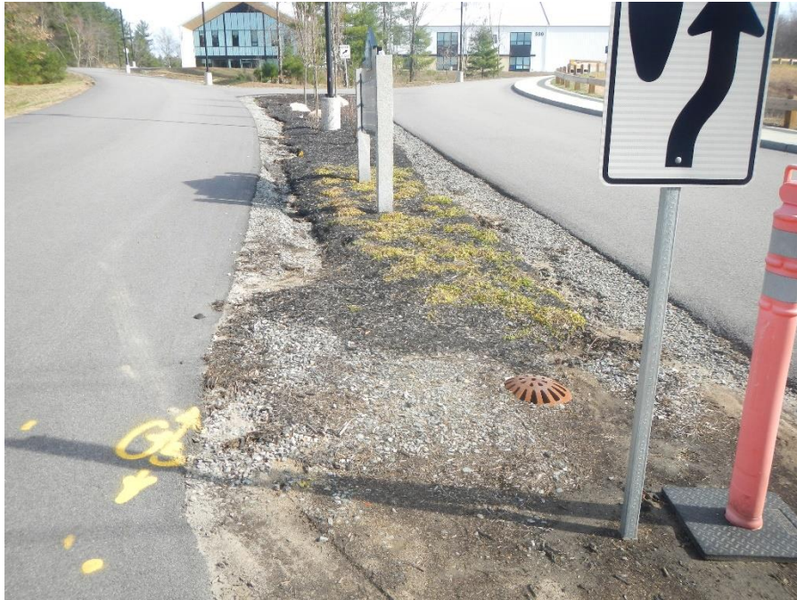
Erosion and sedimentation near catchment structure. Flow may bypass onto Financial Way
