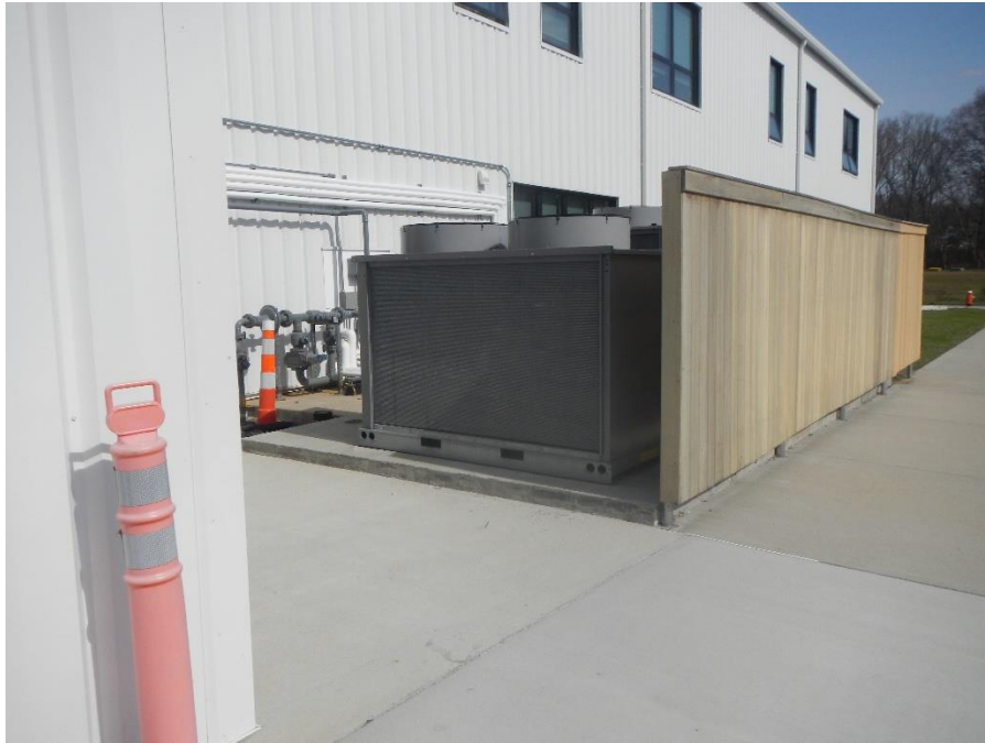
Equipment area located off accessible walkway near gymnasium
