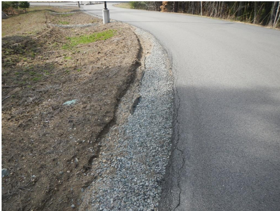
Erosion located adjacent to swale
