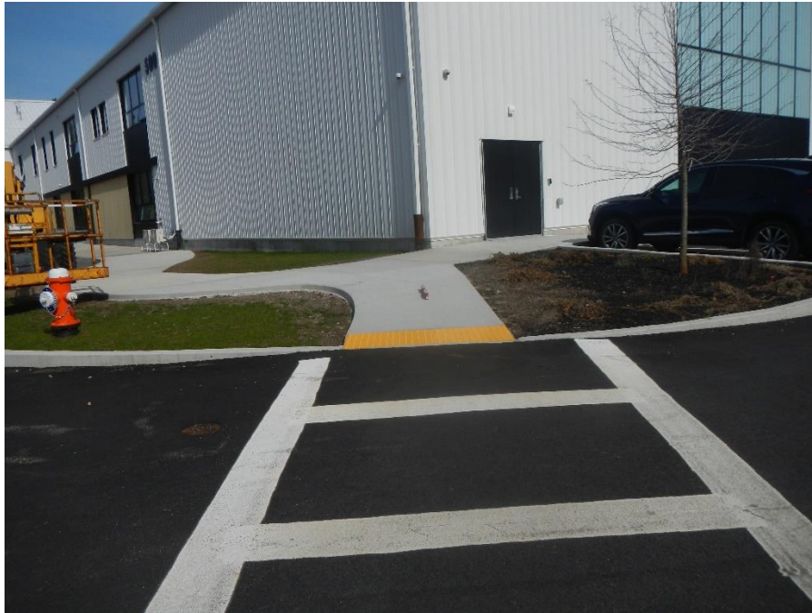
Accessible ramp which appears to require handrails, loam needs to bring landscape area to grade
