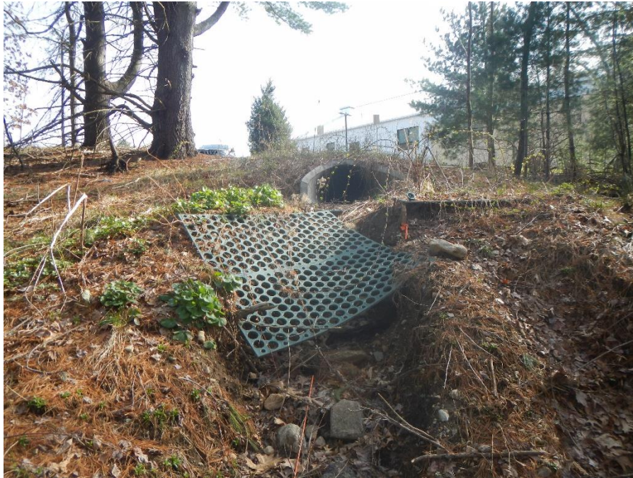
Significant erosion at easterly outfall
