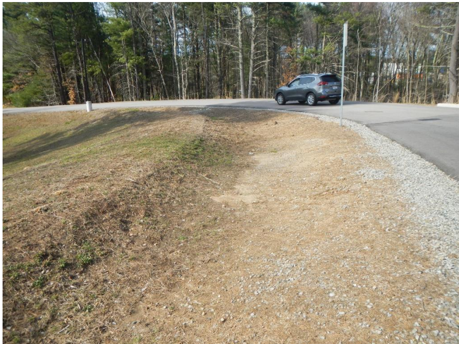
Stormwater swale lacking vegetation, some damage to adjacent pavement (not pictured).
