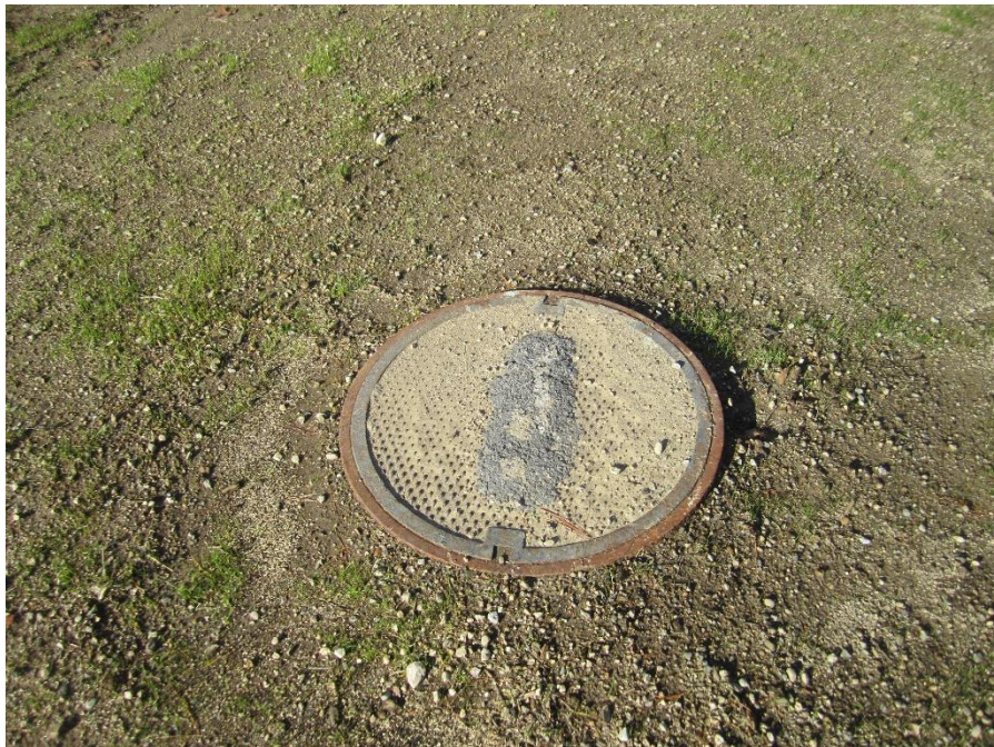
Manhole cover with bituminous patch over lettering
