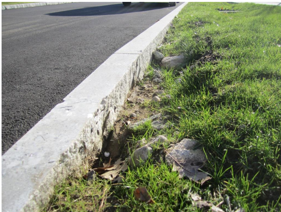
Small area of erosion behind curb line
