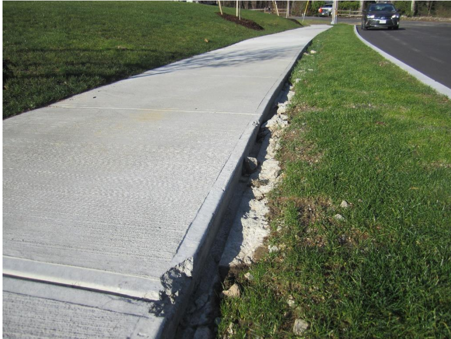
Small area of erosion adjacent to sidewalk
