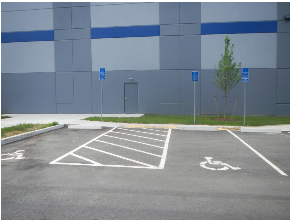
Revised accessible parking location (photo taken prior to access aisle modification to meet ADA)
