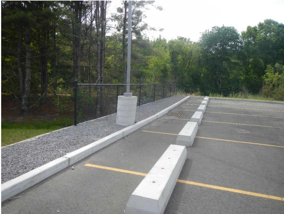
Heavy duty car stops added to truck parking area on south side of site
