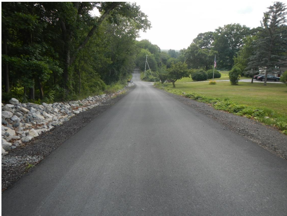
Paved section of Spring Street with dense grade shoulder and rip rap swale
