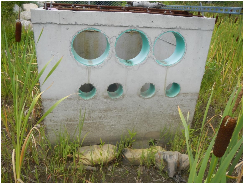
Sandbags that require removal from Infiltration Basin 1 outlet control structure
