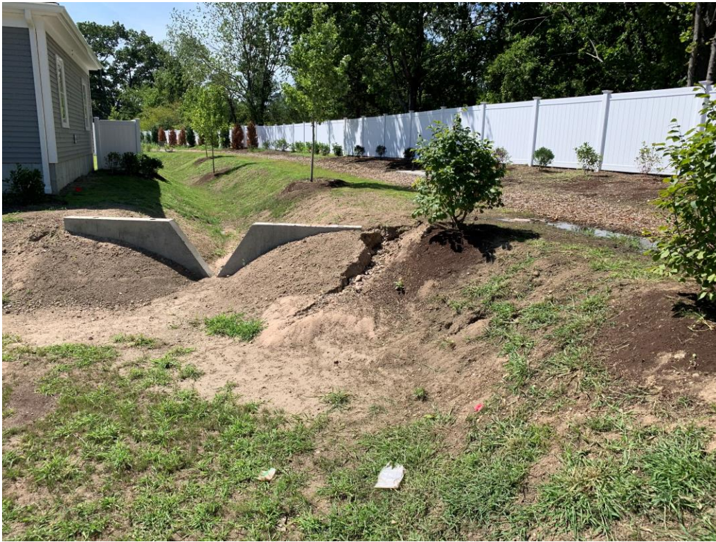
Erosion along the westerly slope of Sediment Forebay 2
