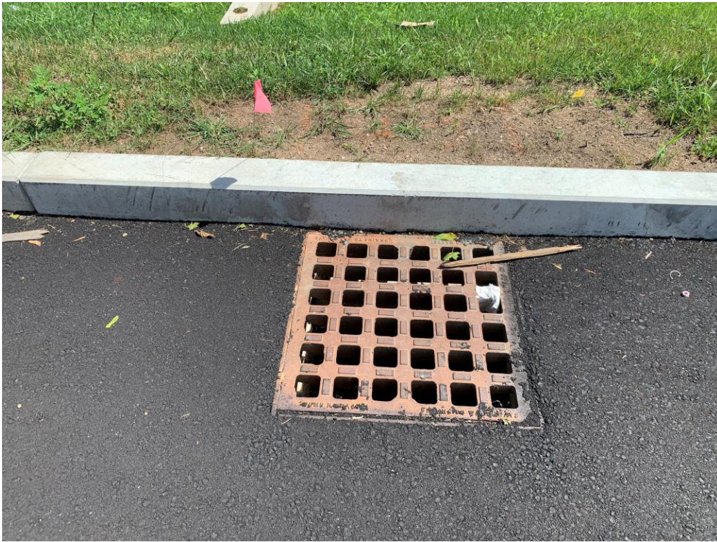
Curb inlet stones have not been installed
