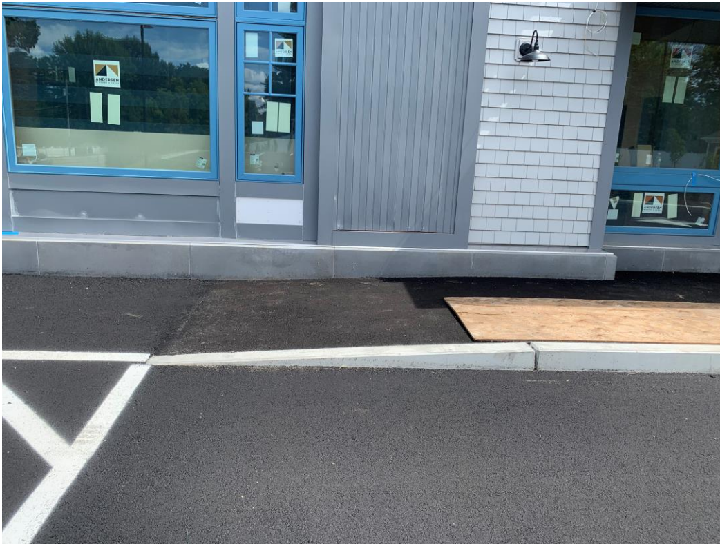
Typical transition curb and bit ramp on the Western side of the Community Bldg.
