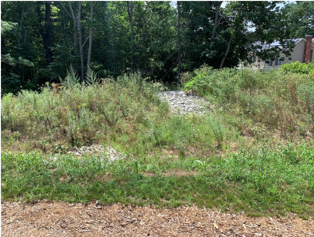
Overgrowth present in Infiltration Basin 3
