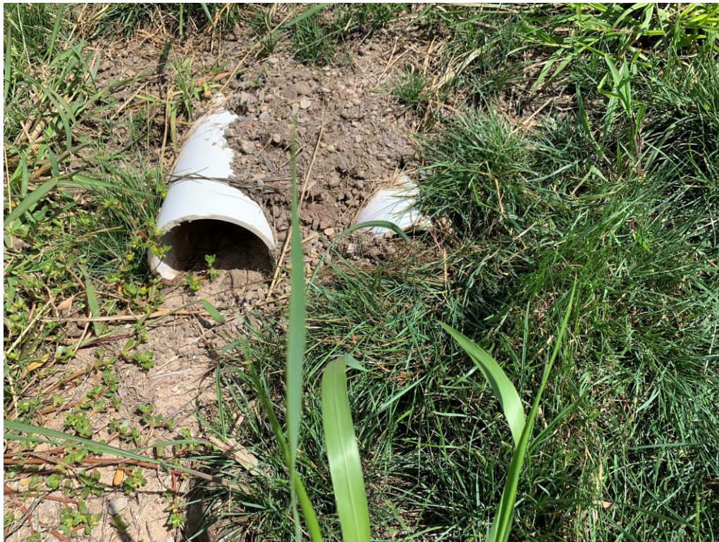
Clogged Roof Drain coming into Infiltration Basin 2
