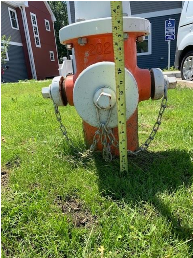
Hydrant in front of Unit B will need to be raised
