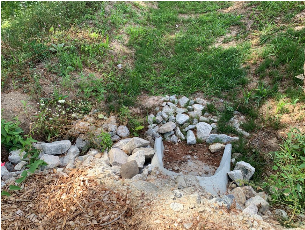
Additional Rip Rap should be installed at the Drainage Swale at the rear of the site
