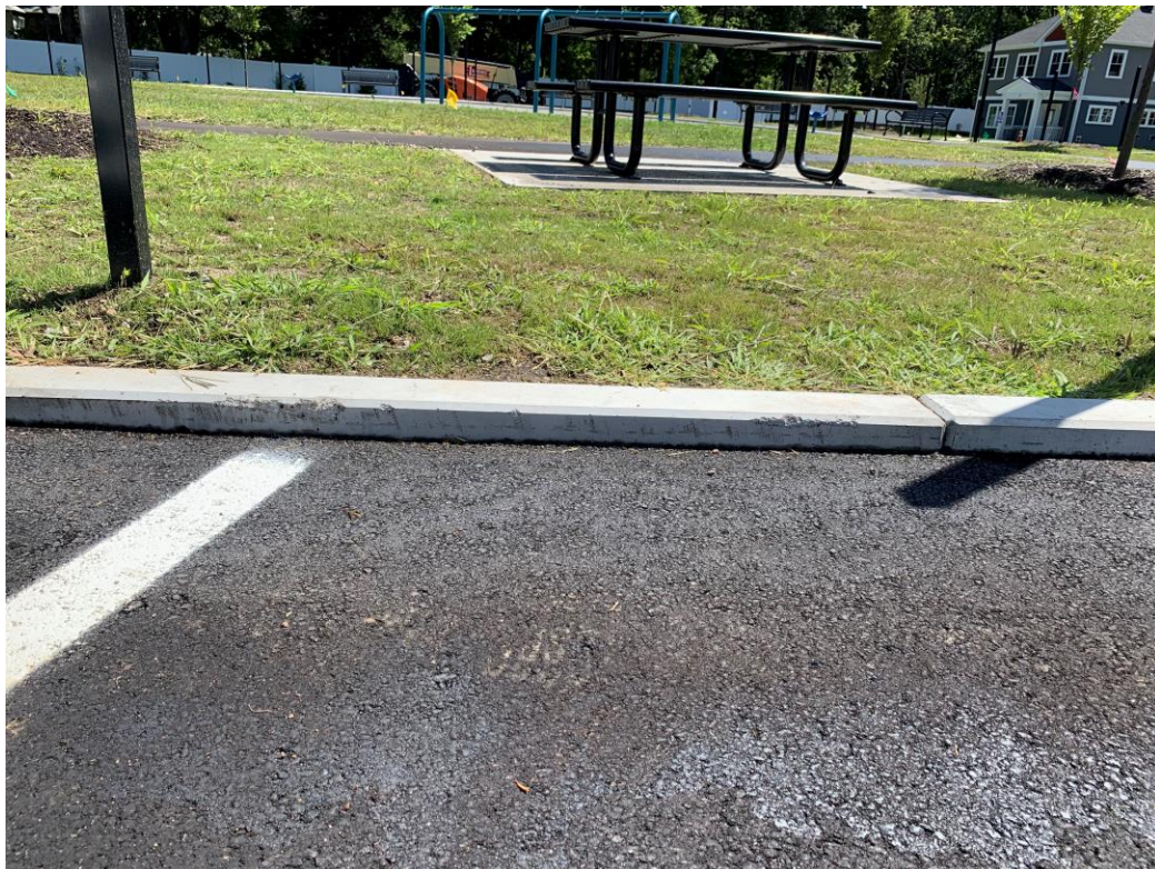
Minimal curb reveal between parking and the westerly side of the Common Area
