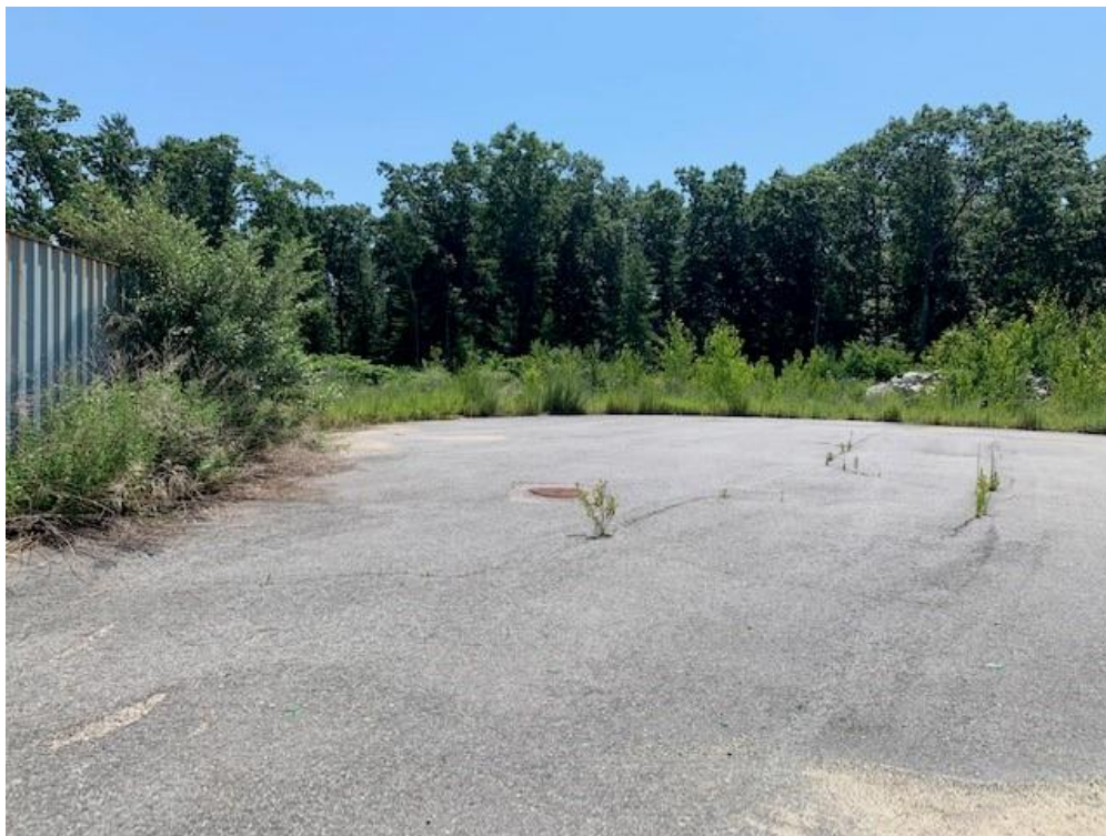
Typical cracking in the cul-de-sac pavement
