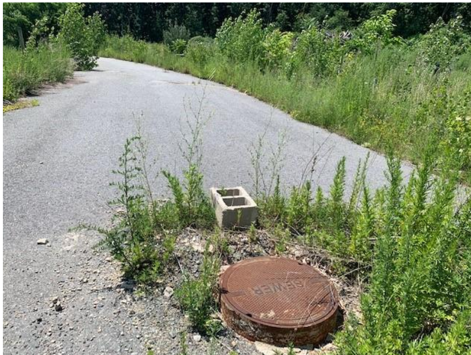
Typical pavement damage adjacent to SMH 1A, which will require repair.
