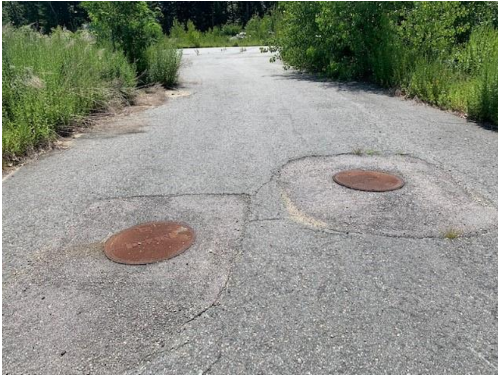
Typical pavement distress
