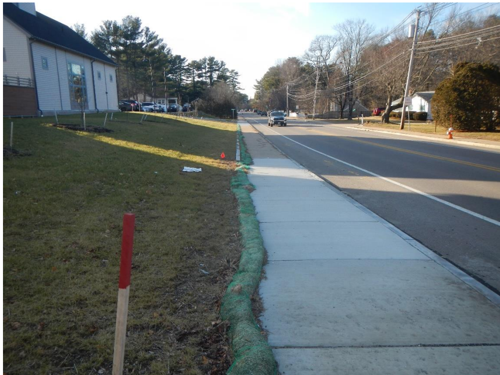
Erosion controls that require removal
