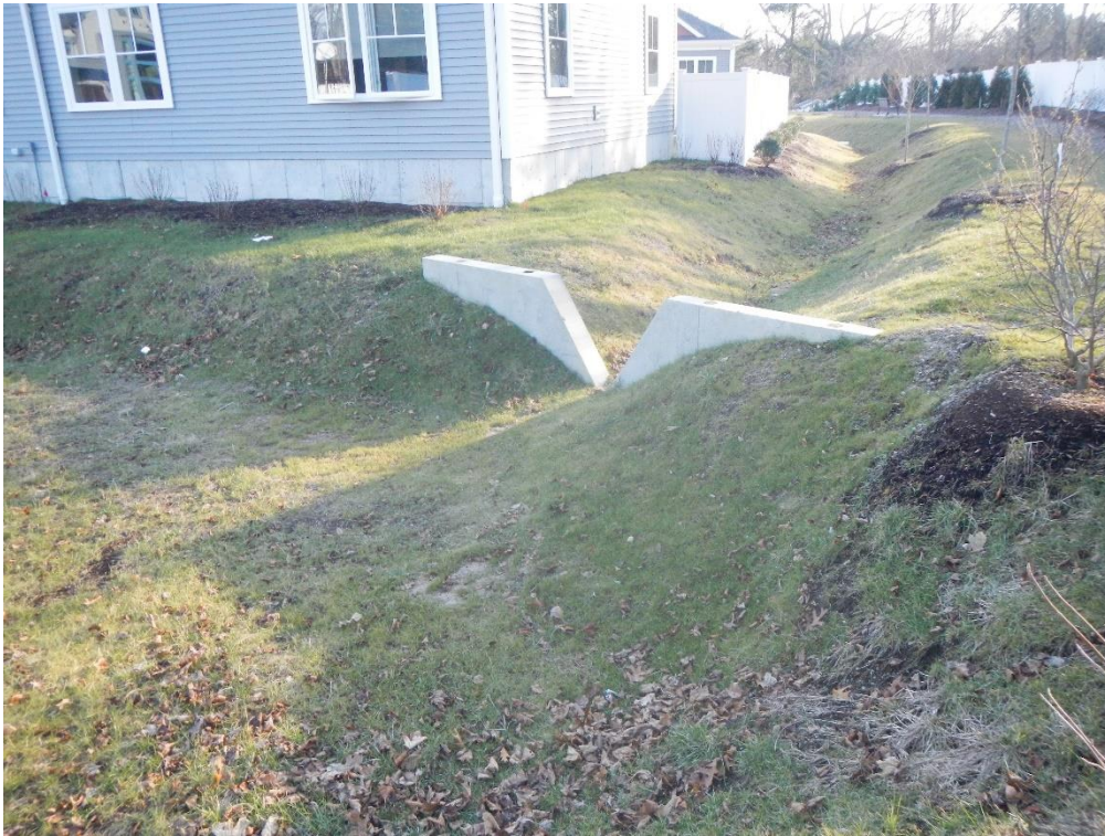
Area of repaired erosion (at concrete weir)
