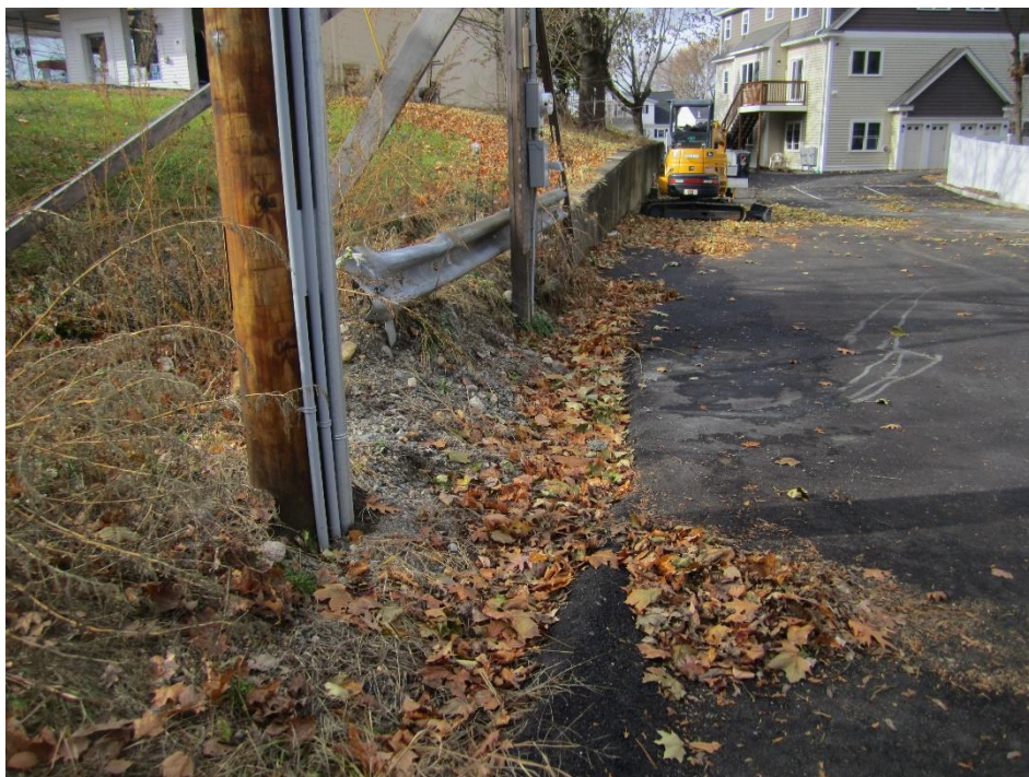
Area between retaining wall and street line that lacks curb installation (photo 11/11/20)
