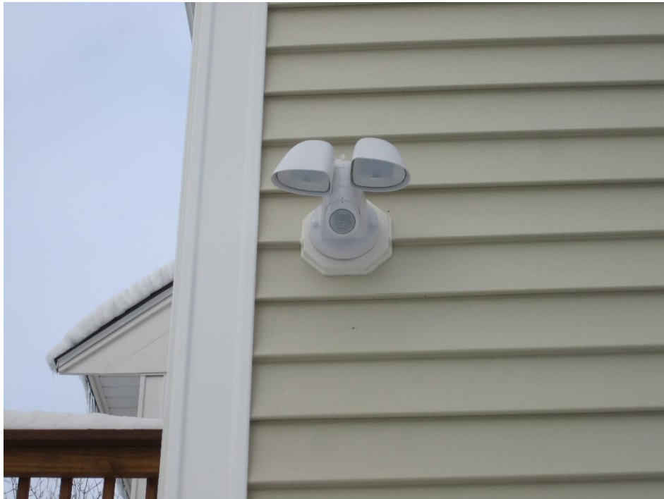
Light fixture at southeast corner of building mounted approx. 12 feet above ground (photo 02/04/21)
