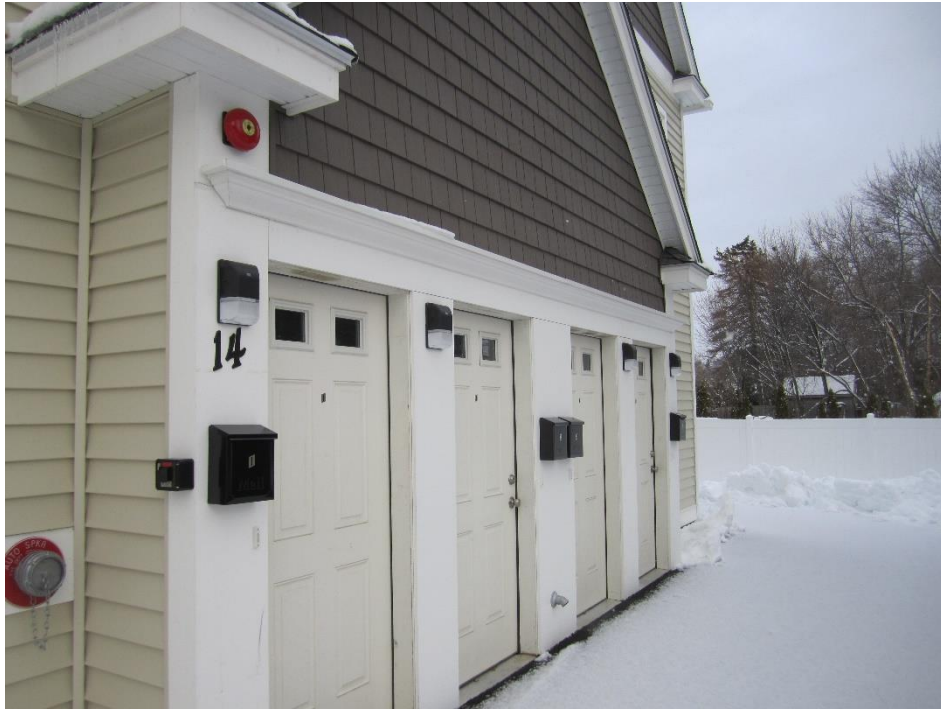
Typical sconce lighting at entryways
