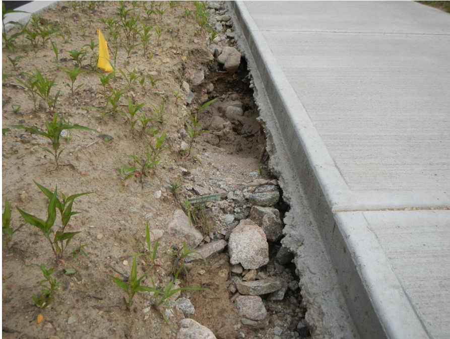
Erosion beginning to undermine sidewalk
