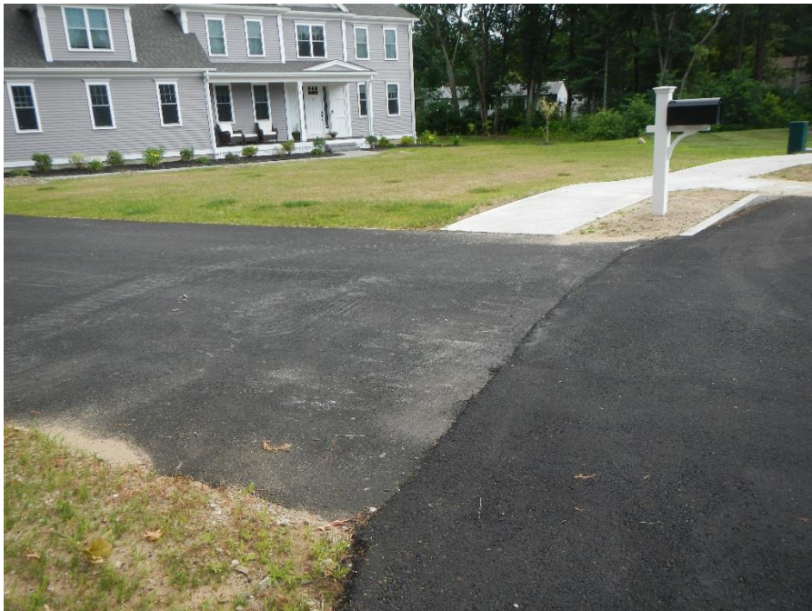
Driveway that lacks 2' granite radius stones
