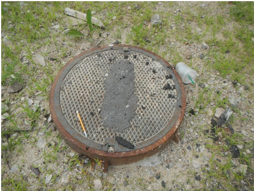
Manhole cover with bituminous patch over lettering
