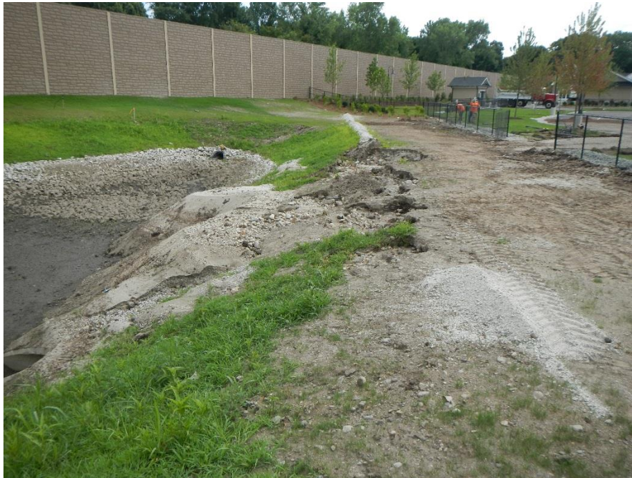
Sediment Forebay 1A that requires slope repair
