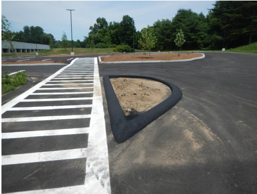
Landscape island formed with cape cod berm set on top course pavement
