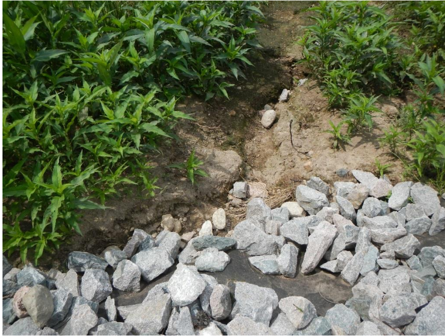
Some erosion present from sediment forebay overflow into infiltration basin
