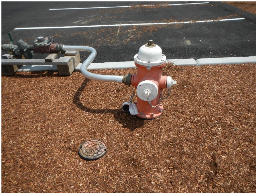
Hydrant that does not appear to be factory painted and is set low for hydrant wrench operation
