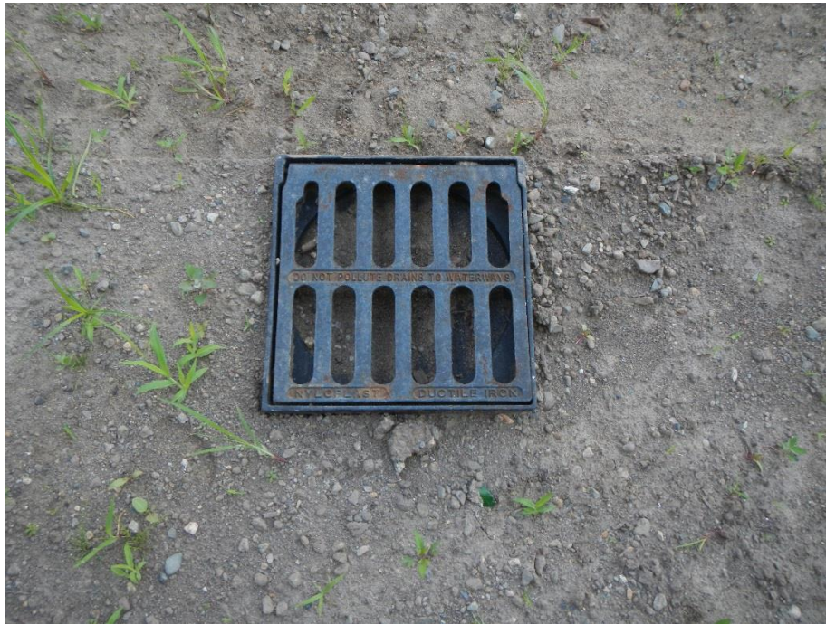
Area drain at Building 3 filled with sediment
