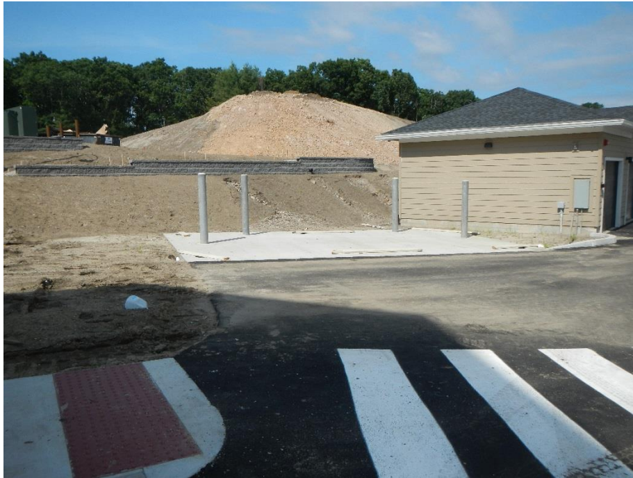
Typical dumpster area that requires completion
