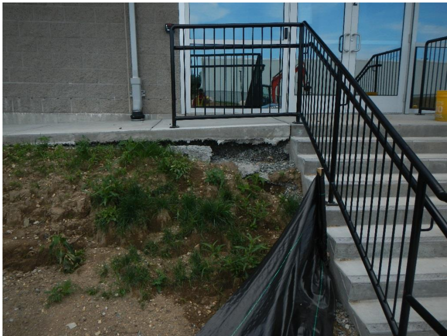
Sidewalk area that is undermined
