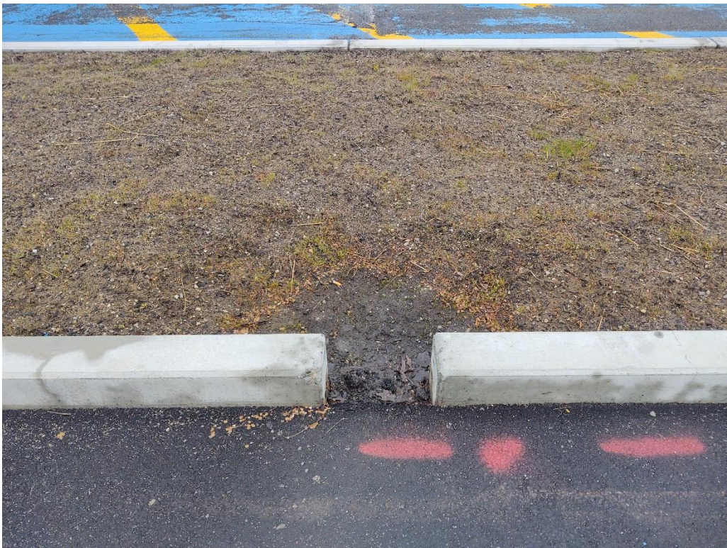
Bioretention area that requires regrading
