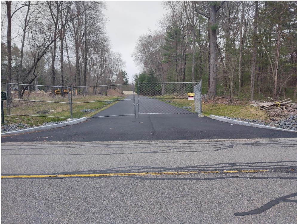
Roadway entrance with temporary construction fence
