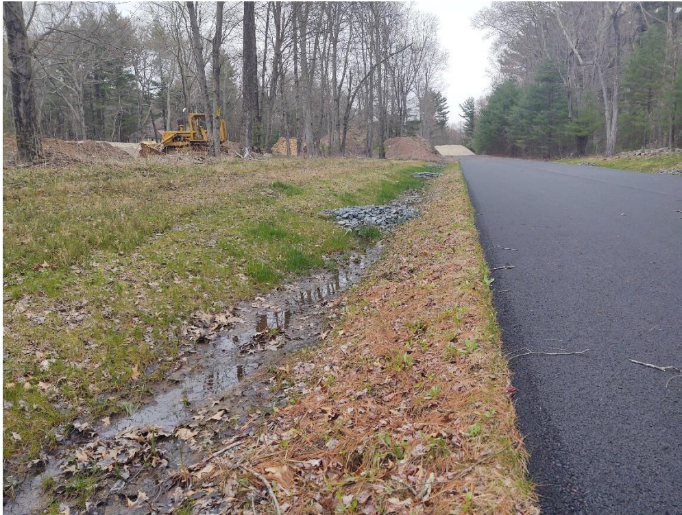
Typical drainage ditch with stone check dams
