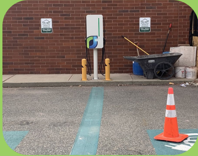
EV Charger #1 - Town Hall
