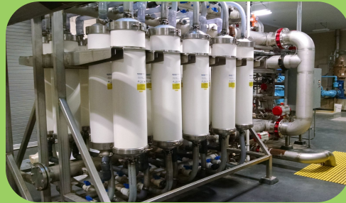
Hayward Water Treatment Plant
