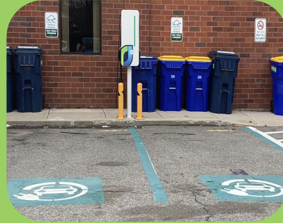
EV Charger #2 - Town Hall
