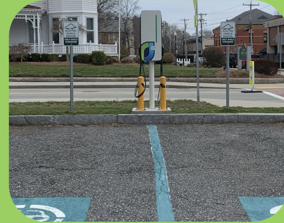
EV Charger #4 - Library
