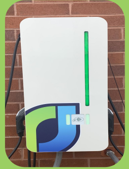
EV Charger #3 - Town Hall
