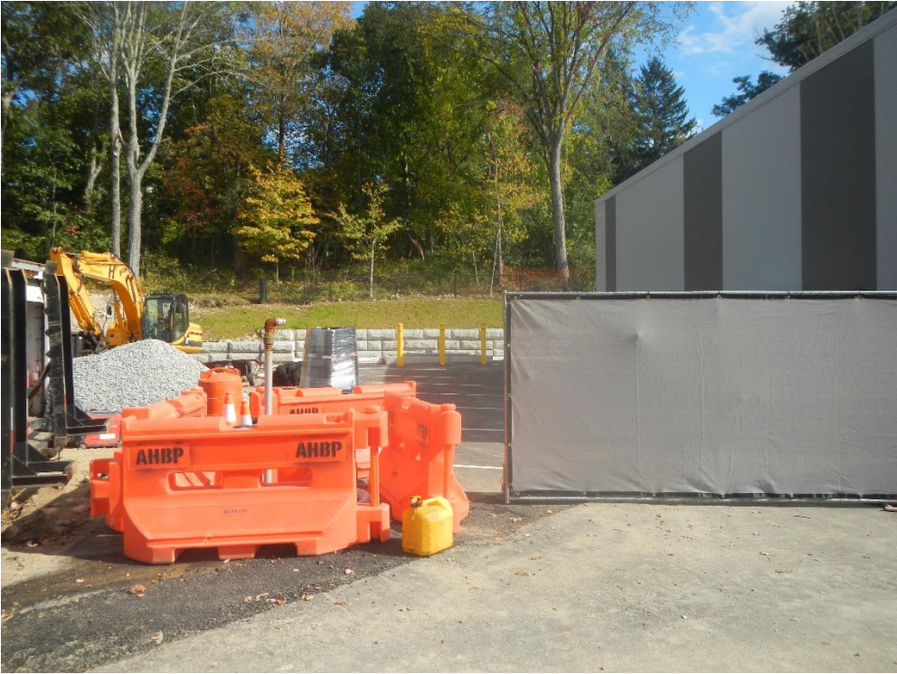
Paved area north of Building 1 with gated access being used for storage
