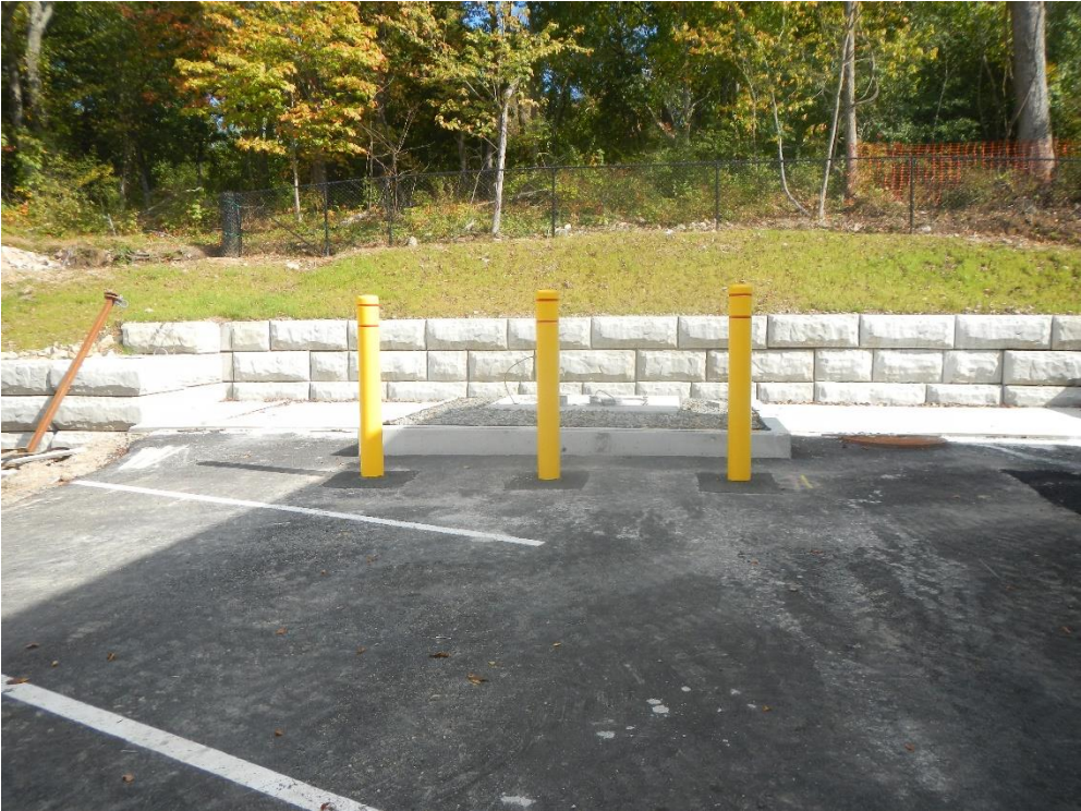
Future transformer location (center) and dumpster pad (left) with minimal pavement access
