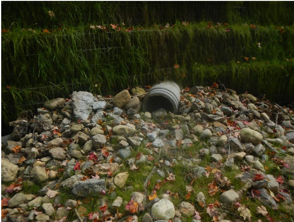
Partially blocked drainage outlet lacking flared end section and with reduced area of rip rap
