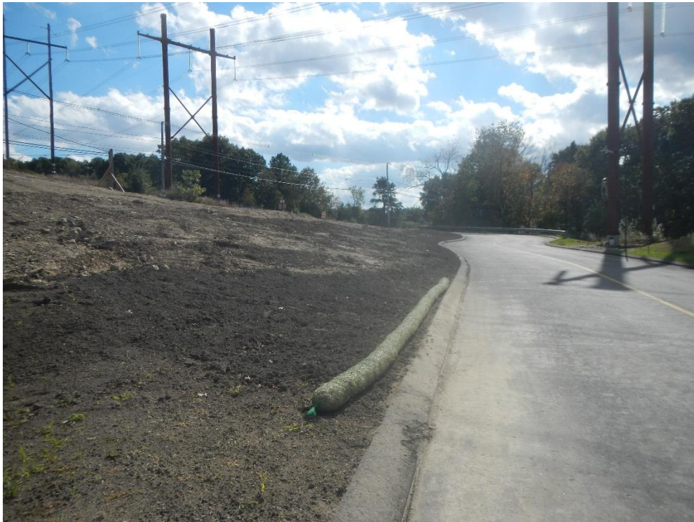
Unstabilized slope with insufficient erosion and sedimentation controls
