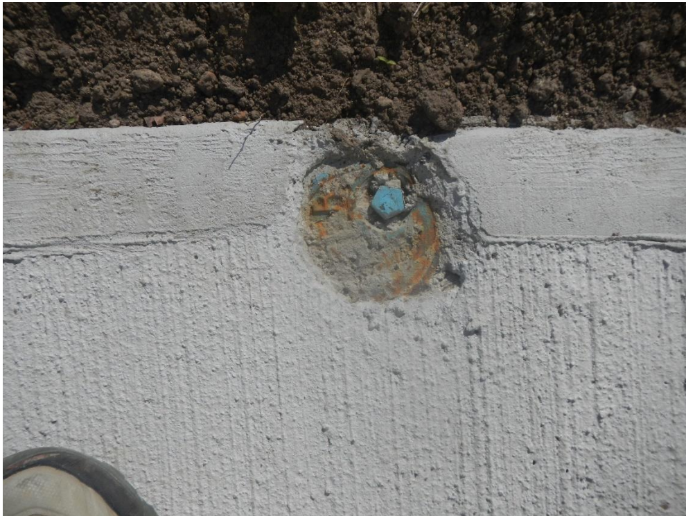
Water curb stop within sidewalk
