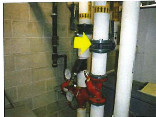
Valve & Fitting Insulation – the butterfly valve at the pumps needs to be insulated in order to reduce distribution losses (West Central St Fire Station).
