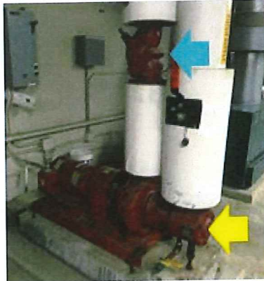
Valve & Fitting Insulation – the suction diffuser (yellow) and strainer (blue) are not insulated which is leading to unnecessary distribution losses (Keller Sullivan School).
