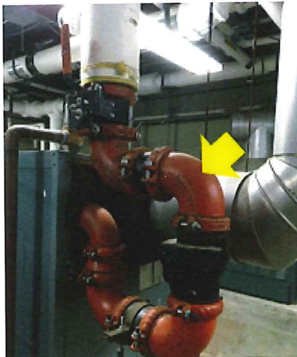
Pipe Insulation – Victaulic pipe insulation was removed. Exposing pipe to unconditioned boiler room is leading to unnecessary distribution losses (Keller/Sullivan School).
