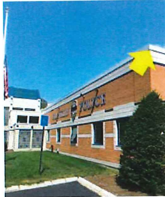
Roof-Wall Intersection Air Sealing – the exterior flashing and finishes at the roof-wall intersection are not constructed to stop air leakage (Police Station).
