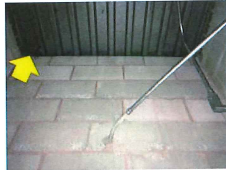
Roof-Wall Intersection Air Sealing – gaps between the roof deck and the wall framing are pathways for unwanted infiltration/ exfiltration (Police Station).
