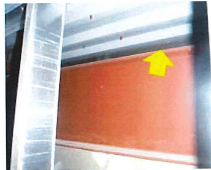
Roof-Wall Intersection Air Sealing – gaps at the interior of the roof-wall intersection combine with the unsealed exterior flashing and finish details to allow unwanted infiltration/ exfiltration (Municipal Building).
