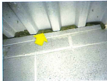
Roof-Wall Intersection Air Sealing – fiberglass was used to fill gaps between the roof and wall framing components. Fiberglass is an air permeable material that needs to be covered with an air barrier to avoid further air leakage at the roof-wall intersection (Keller Sullivan School).
