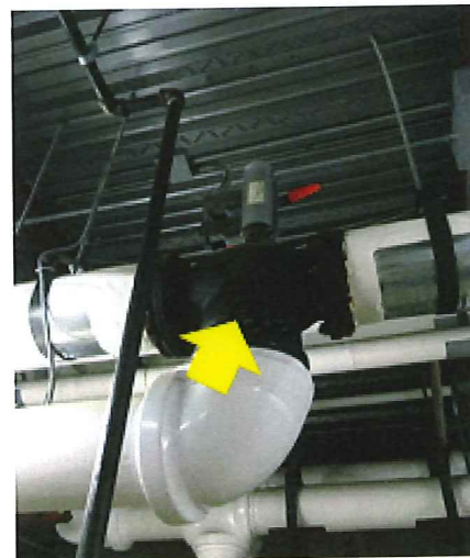
Valve & Fitting Insulation – the 3-Way valve in the distribution system is a tricky component to insulate. The large uninsulated surface needs to be wrapped in order to reduce distribution losses (Keller Sullivan School).
