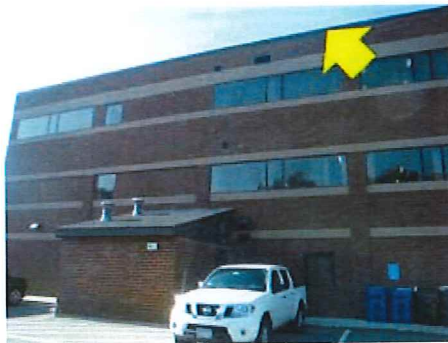
Roof-Wall Intersection Air Sealing – the exterior flashing and finishes at the roof-wall intersection are not constructed to stop air leakage (Municipal Building).
