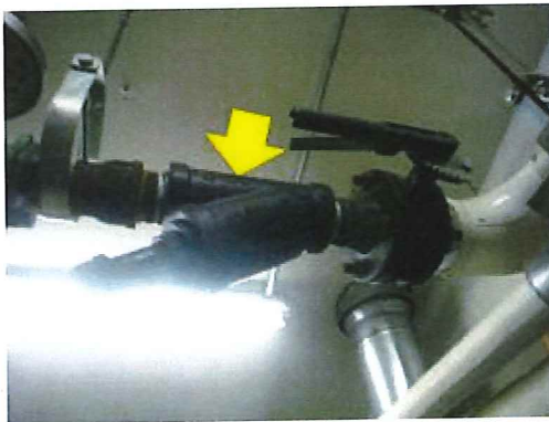
Valve & Fitting Insulation – the strainer is uninsulated which is leading to unnecessary distribution losses (Municipal Building).
