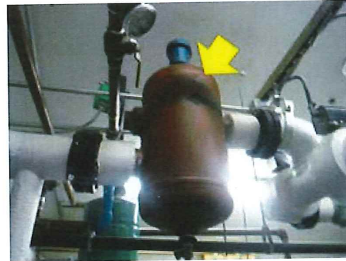
Tank Insulation – the air separator tank represents a large surface area in the heating distribution which if continued to left uninsulated will result in distribution losses (Municipal Building).
