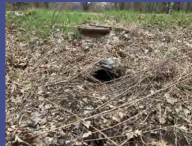
4/6/2021 - Lincoln St - debris filled outlet caused overflow and damage to a sidewalk
