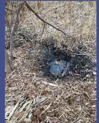
4/12/2021 Highland St clogged outlet
