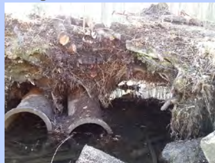
Culvert under the Beaver St interceptor (24" sewerline) on the verge of collapse - 2014
